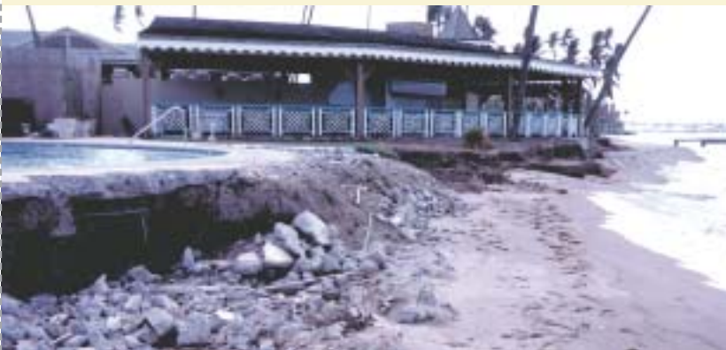
Pinney's Beach, October 1995, after Hurricane Luis
