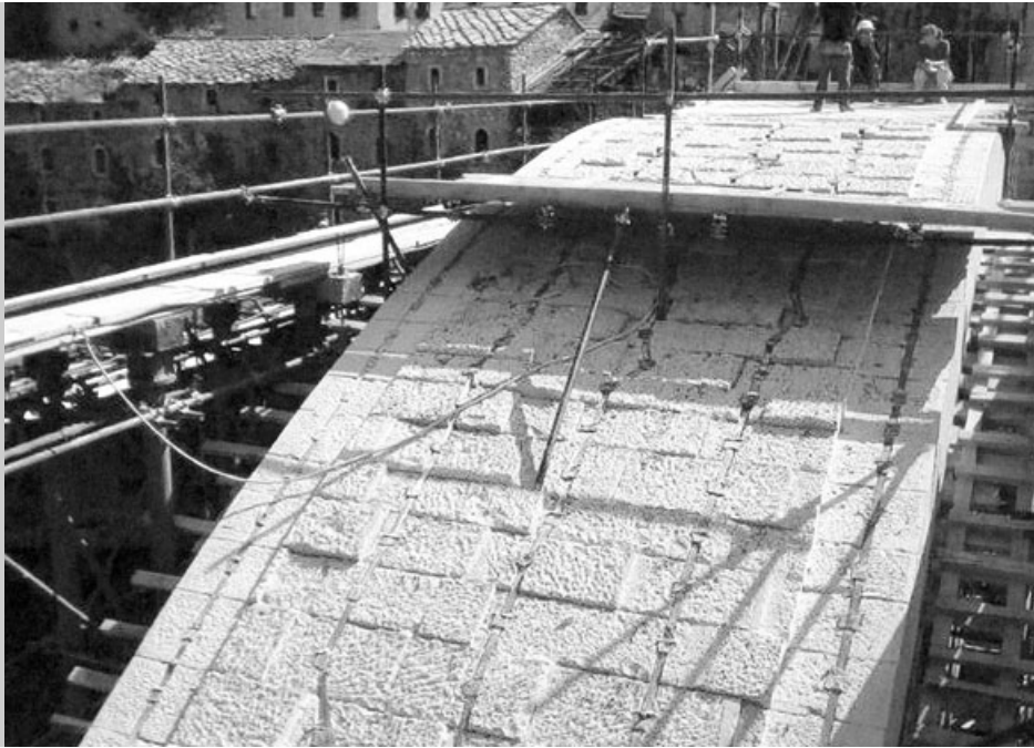
8. The new arch of the bridge reconstructed with the original technique using stainless steel.
