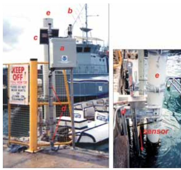
Rarotonga sea level station, Avarua Harbor, Cook Islands. The fiberglass electronics package (a), antenna (b), solar panel (c) were installed on a pier. Conduit (d) containing cables connecting the sensor, located at a depth of five feet below low-tide water level, to the data collection platform containing the electronics above, was externally attached to the tube containing the sensor (e).
