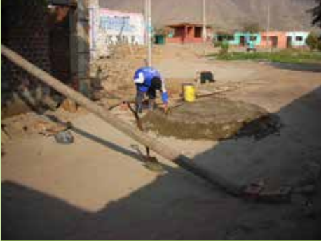
Figure 3.2.9. Concrete mixing on ground on site Mixing is carried out without sheets or others tools
