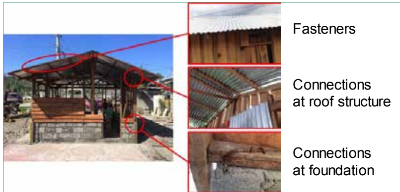
Figure 1. A non-engineered construction (left) and identified weak points by field survey (right).
