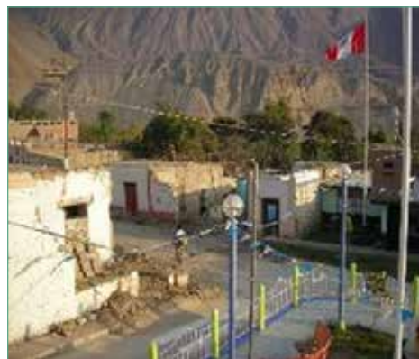
Figure A.2.6 Collapsed houses in central area of Zuniga, Lima state
