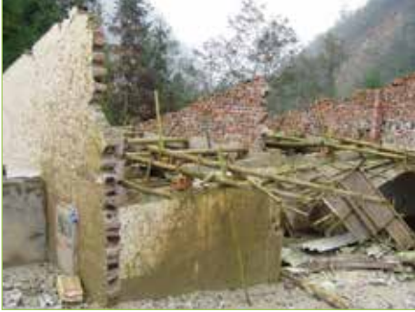
Figure 3.1.18. Damaged brick house
