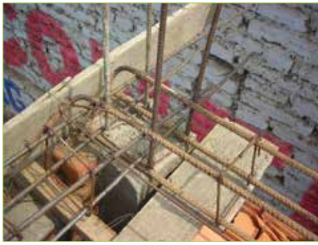
Figure 3.2.12. Corner of beams and column Length of lapped splices is limited to the dimension of RC members' section size because of fabrication method
