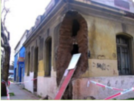
Figure 3.1.9. Damaged adobe construction in Santiago
