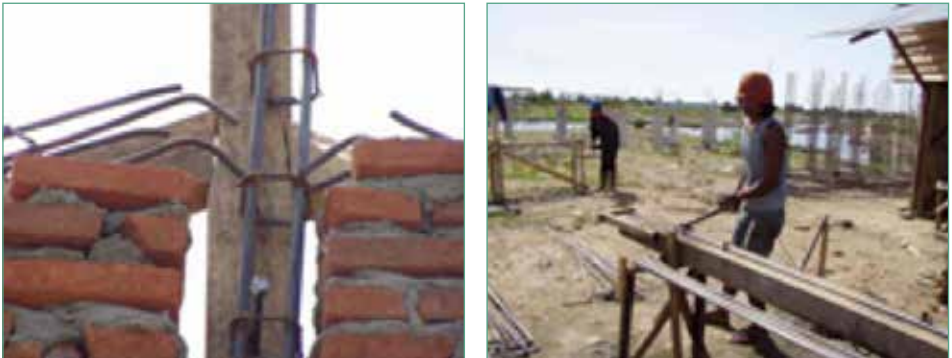
Figure 1.1.5 Inadequate detailing of rebar connections (left), and bending of rebar on site with simple tools (right), in Banda Aceh, Indonesia
