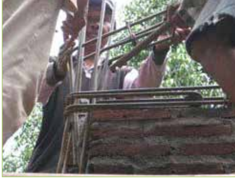
Figure 3.2.18. Connection of RC members Horizontal rebar for beams is not connected at the corner
