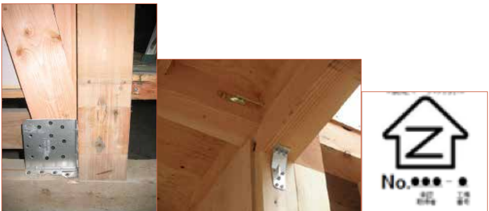
Figure 5.4.6 Example of metal connectors. Brace to plinth/column type (left), column to beam type (middle) Certificate mark of quality assurance scheme (right)
