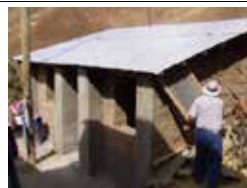
A seismic adobe house being constructed in the rural area development project by the NGOs
