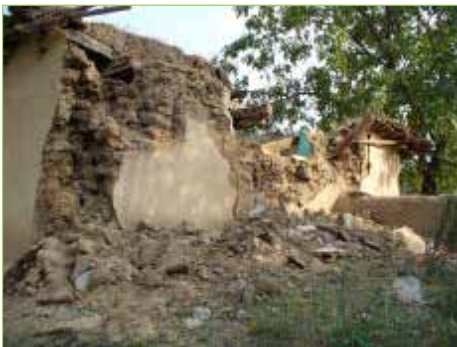
Figure 3.1.24. Adobe house damaged by the earthquake
