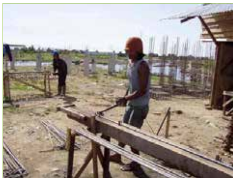
Figure 3.2.7 Bending works on site with simple tools Assembling of rebar is also conducted on ground
