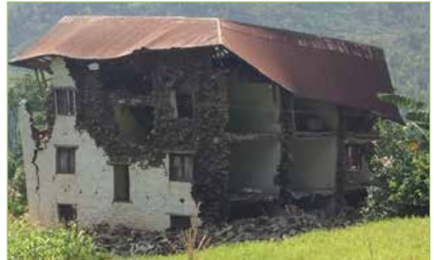
Figure 3.1.7. Delamination of masonry walls
