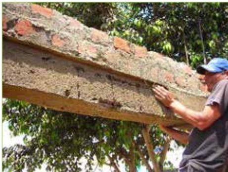
Figure 3.2.14. Honey comb in beam Some of rebar is exposed to air observed
