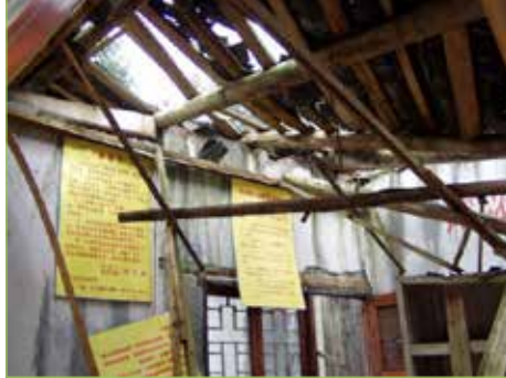
Figure 3.1.19. Collapsed building due to failure of gable wall
