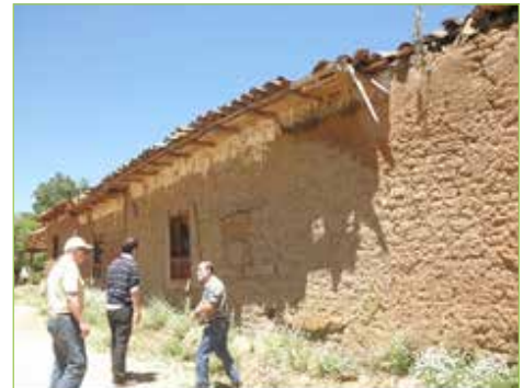
Figure 3.1.12. Adobe construction without appropriate maintenance work in Huerta del Maule in Maule Region
