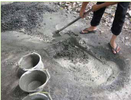
Figure 3.2.15. Concrete mixing on ground on site Mixing is carried out without sheets or other tools
