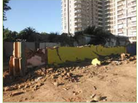
Figure 3.1.10. Damaged adobe construction located next to undamaged high-rise building in Talca
