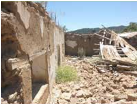
Figure 3.1.11. Damaged adobe construction in Nirihiulo in Maule Region
