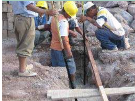
Fig. A.2.2 Construction of a model house by participants under technical guidance of experts
