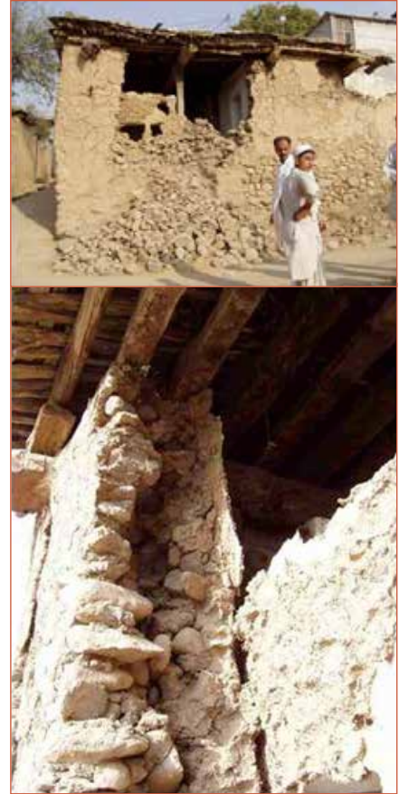
Figure 5.2.3 Typical damage to houses of undressed stone masonry with mud mortar, as shown in the Guideline (2005 Northern Pakistan Earthquake (Kashmir Earthquake)) Much typical damage to various types of structures are addressed
