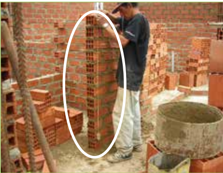
Figure 3.2.11. Laying work of bricks with plumb bob Taut line is usually used
