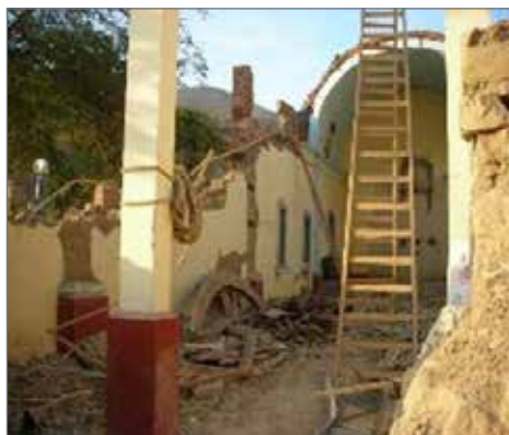
Figure A.2.5 Heavily damaged church (Adobe wall, vaulted roof made from quincha), Zuniga, Lima state
