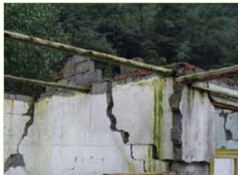
Figure 3.1.17. Damaged concrete block house
