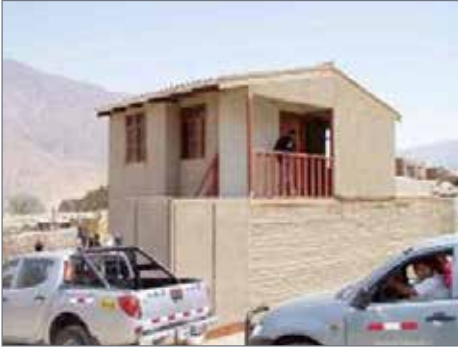
Figure A.2.7 House A: A model house in Zuniga, no structural damage
