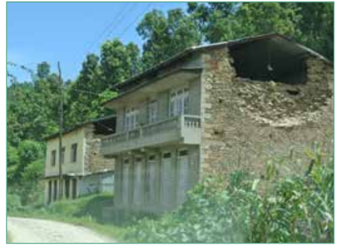
Figure 3.1.5. Out-of-plane failure in masonry walls
