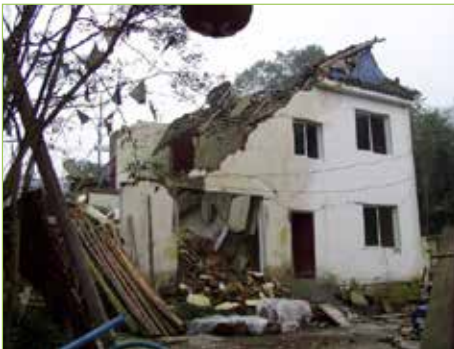
Figure 3.1.14. Damaged house with hollow core slabs PCa
