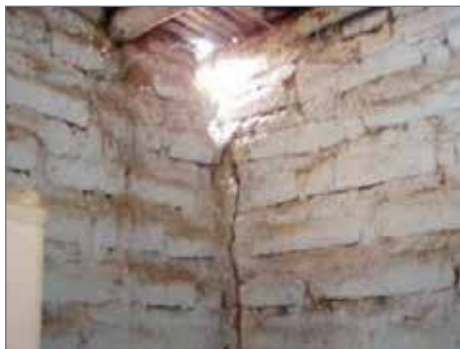
Figure A.2.10 maged Heavy cracks in House B
