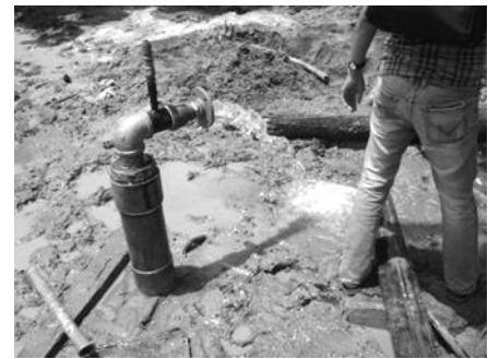
Fig.2 Flowing artesian well in Mae Sai basin, depth of 200 meters with 50-60 m 3 /hour.
