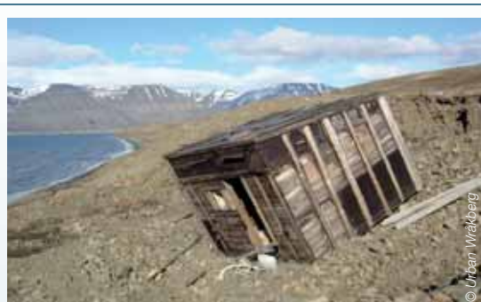
A cabin slides down the erosion edge in Svalbard, which is on Norway's Tentative List for potential World Heritage status.
