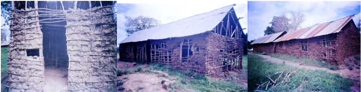
ORIGINAL CONDITION: From right: A makeshift kitchen; classrooms at Bura Primary School
