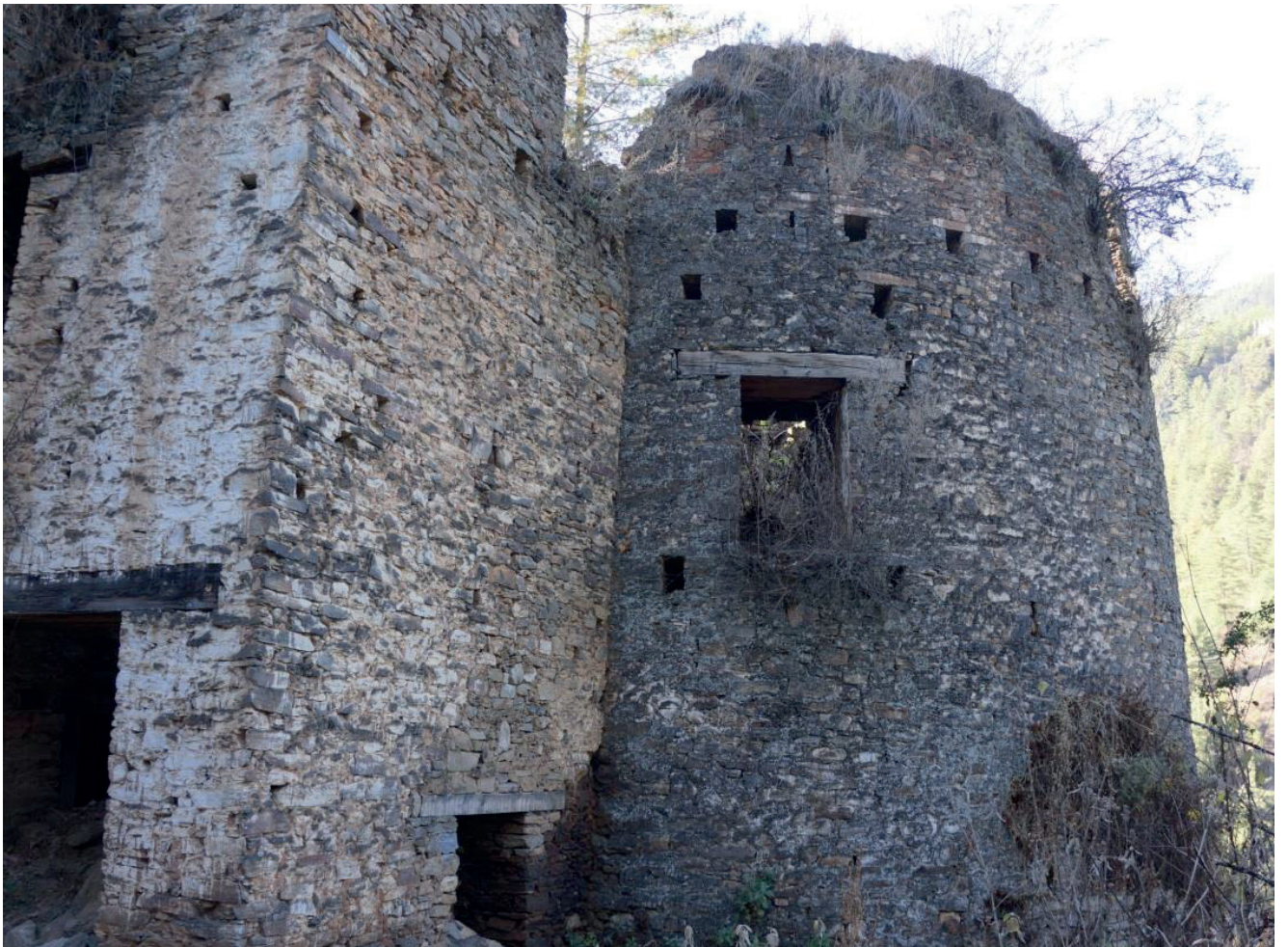
Figure 7. The outer works of Drukgyel Dzong, Bhutan, showing the difficulties of managing this large complex.
