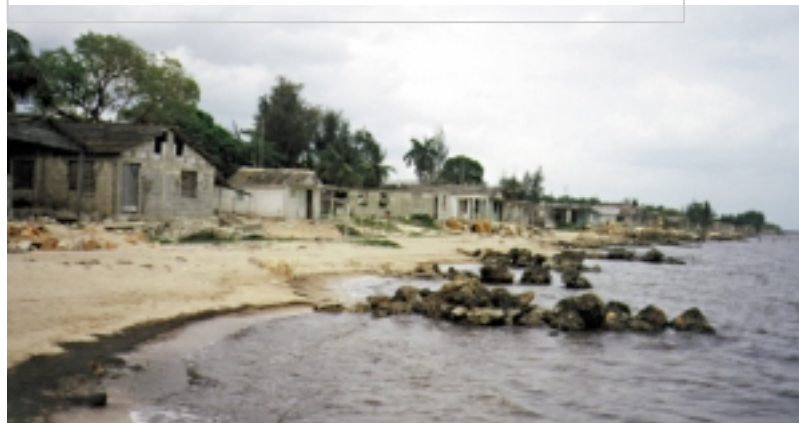
Groynes built by the community to promote beach accretion and protect houses at Playa Mayabeque, Helena del Sur, Cuba, 2001
