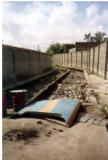
Debris and garbage blocking a drainage channel in Ikoyi Island, Lagos, Nigeria, July 2002.
