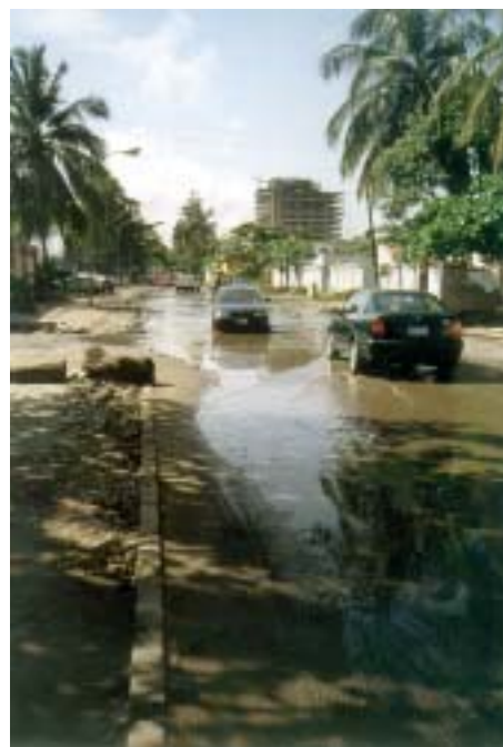
Blocked drainage channels result in frequent flooding during the rainy season, Lagos, Nigeria, July 2002.
