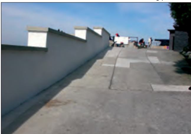
Figure 4. The horrendous supporting wall on the approaches to the Upper Galleries.
