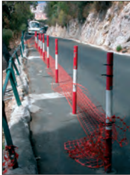
Figure 3. Road works – this makeshift barrier has been present at St. Michael's Cave for over a year, where nothing has been done to improve the situation.
