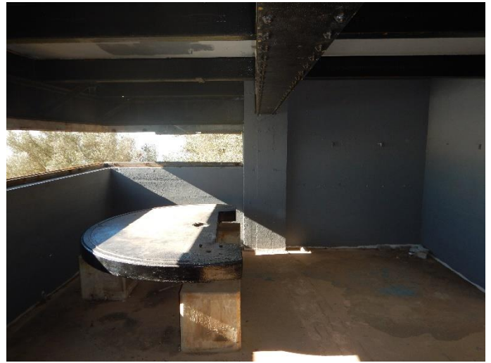
↑ Interior of the Southern Range Finder showing the remaining base of the range finder
