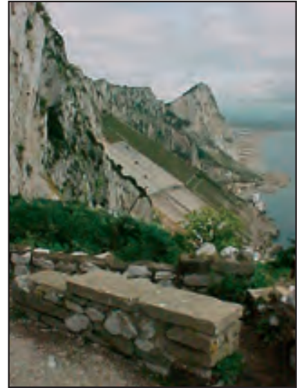
Figure 7. The lookout point that overlooks the eastern side of the Rock is in a state of severe neglect.
