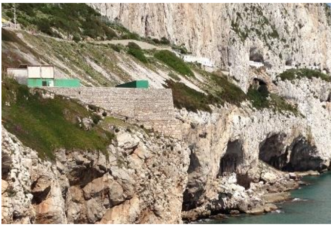
↑Photograph 2: View of 3 rd Europa Advance Battery, from 1 st & 2 nd Europa Advance Batteries before remedial works, showing the sea caves of the candidate World Heritage Site.
