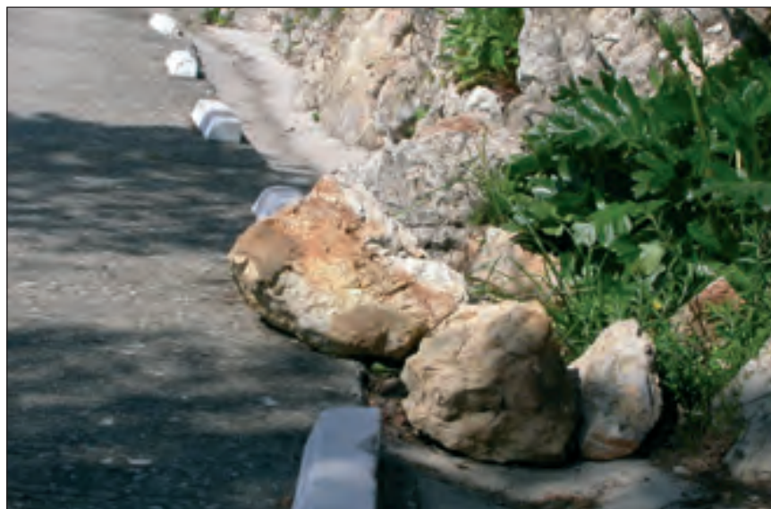
Figure 1. Removal of plants increases soil erosion and leads to rockfalls.
