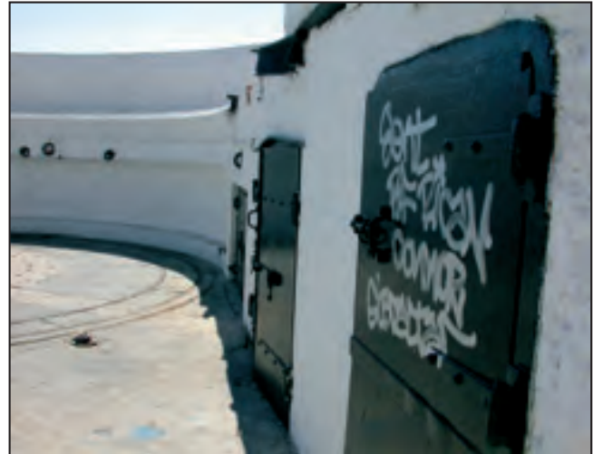
Figure 7. Spur Battery. New graffiti a few months after the site was painted.
