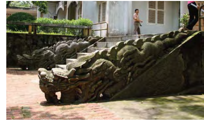
Small dragon stairs with soil level problem — Photo F. Cristofoli, June 2008
