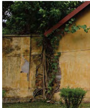
Examples of problems caused by roots: On the pavement — Photo S. Ricca, June 2008 On the masonries — Photo F. Cristofoli, June 2008
