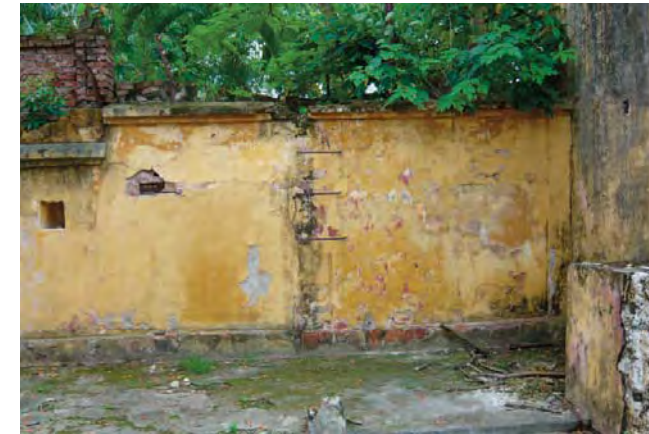
Internal wall of the West gate: gatehouse — Photo S. Ricca, June 2008 Plan of gatehouse — Drawing S. Ricca; June 2008
