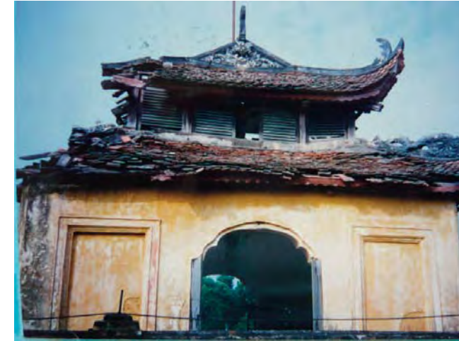
Roof of Hau Lau pavillon before restoration — Department of Culture, Hanoi People's Committee, 1998
