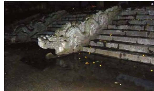
Detail of the cement repairs — Photo F. Cristofoli, June 2008 Problem of water drainage — Photo S. Ricca, June 2008
