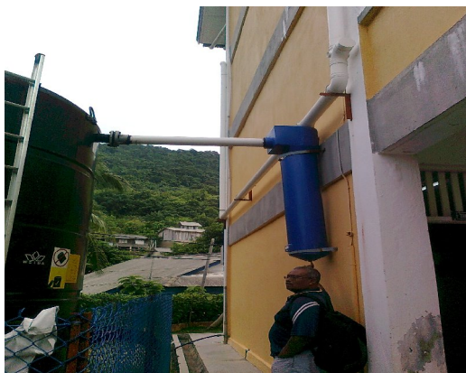
Above Ground Storage Tank (School)
