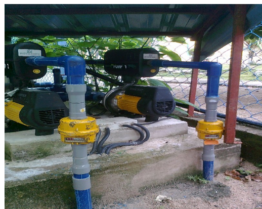
Installed Water Meter for the RWHS
