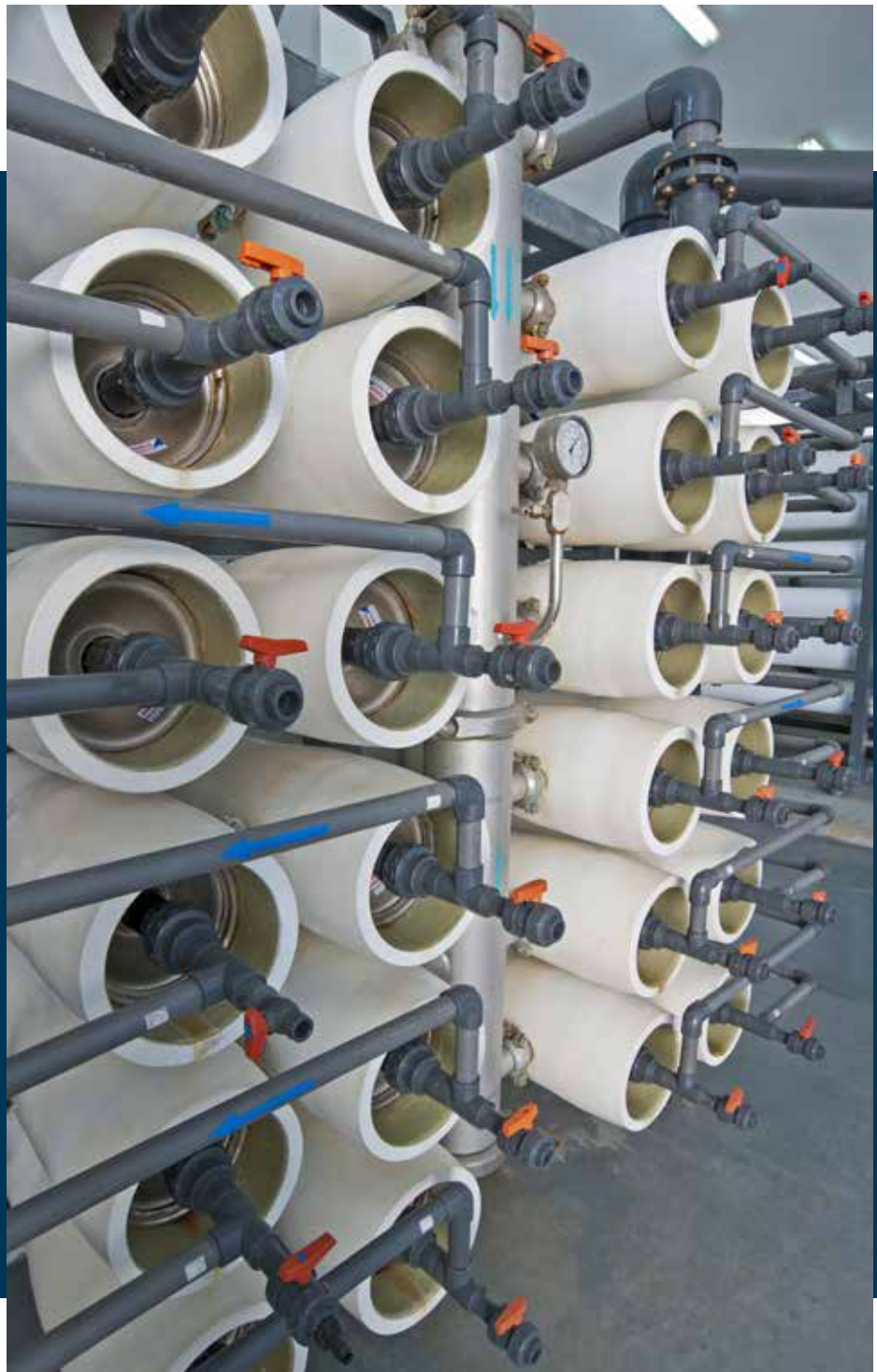
Racks of filters in a desalination plant Photo: © Paul Vinten/Shutterstock.com
