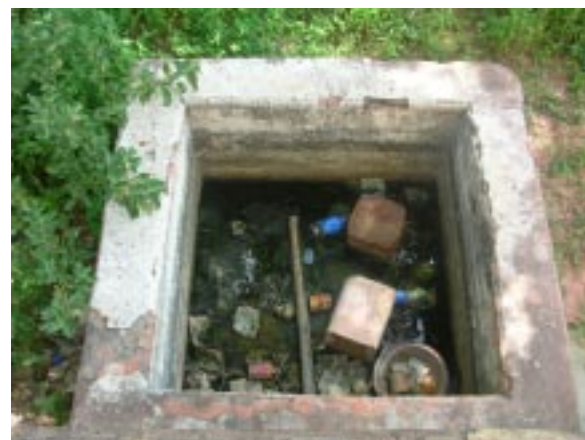
e,f,g,h. Garbage lying around the premises.
