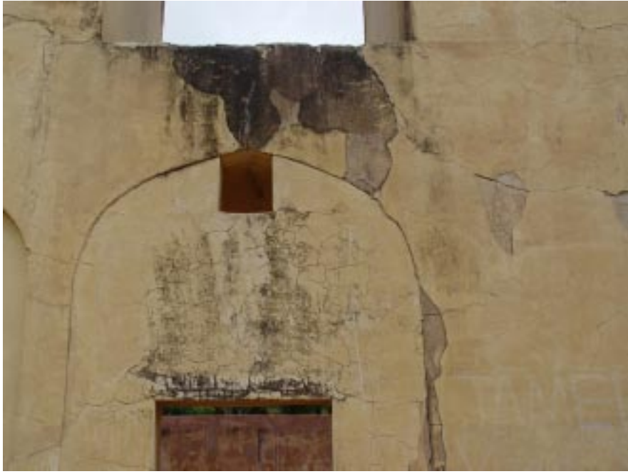
a. An arched opening in the yantra closed and a doorway made to access the portion behind.
