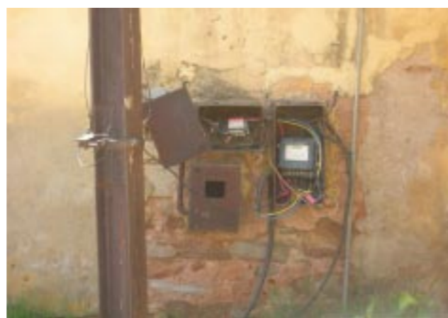
EXPOSED ELECTRICAL METER BOX AND CABLES
