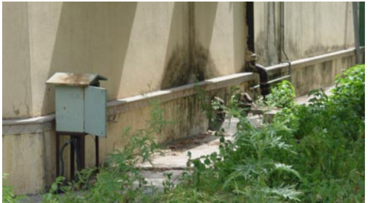
d. Open junction box in the complex.
