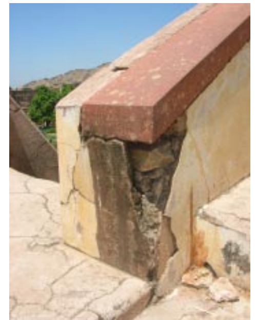
g. Deterioration of the parapet
