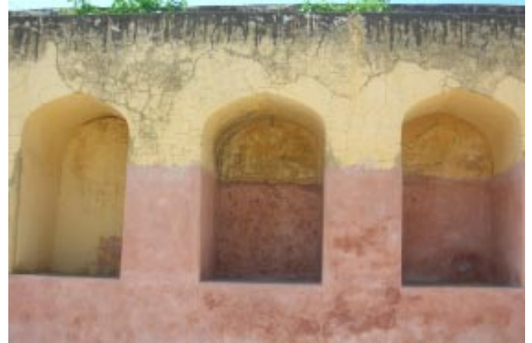
e. Replastering has not been matched with the earlier plaster
