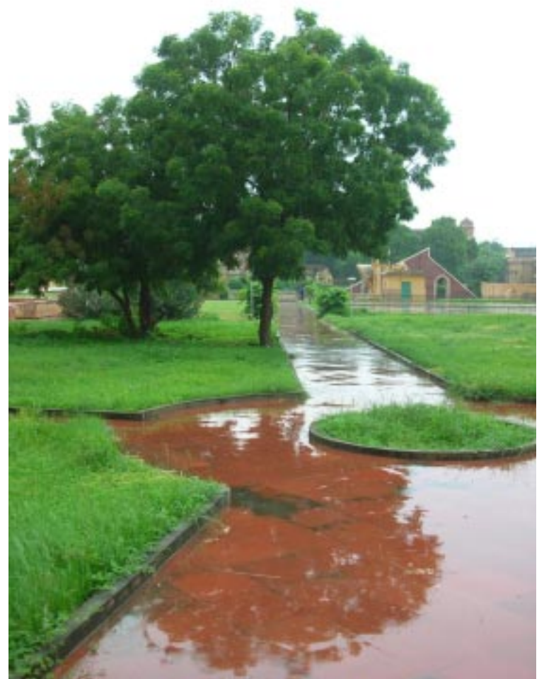
e. Ponding in the pathways will eventually damage them.
