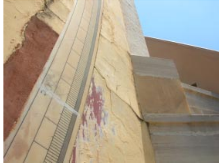
c,d. The repair of the markings has not been done properly
