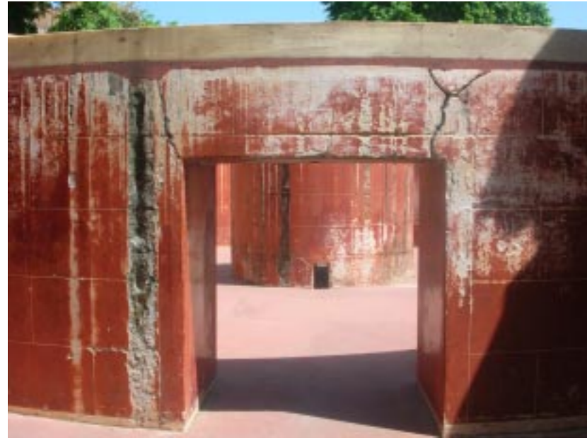
a. The lintels in the Digansha Yantra are cracking and need attention
