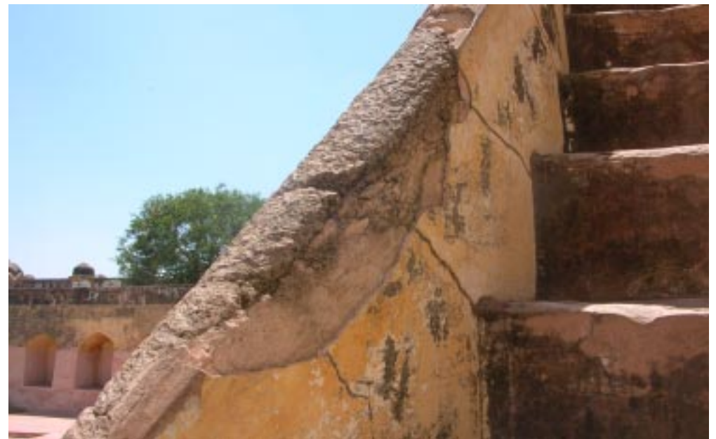
e. Deterioration of the parapet
