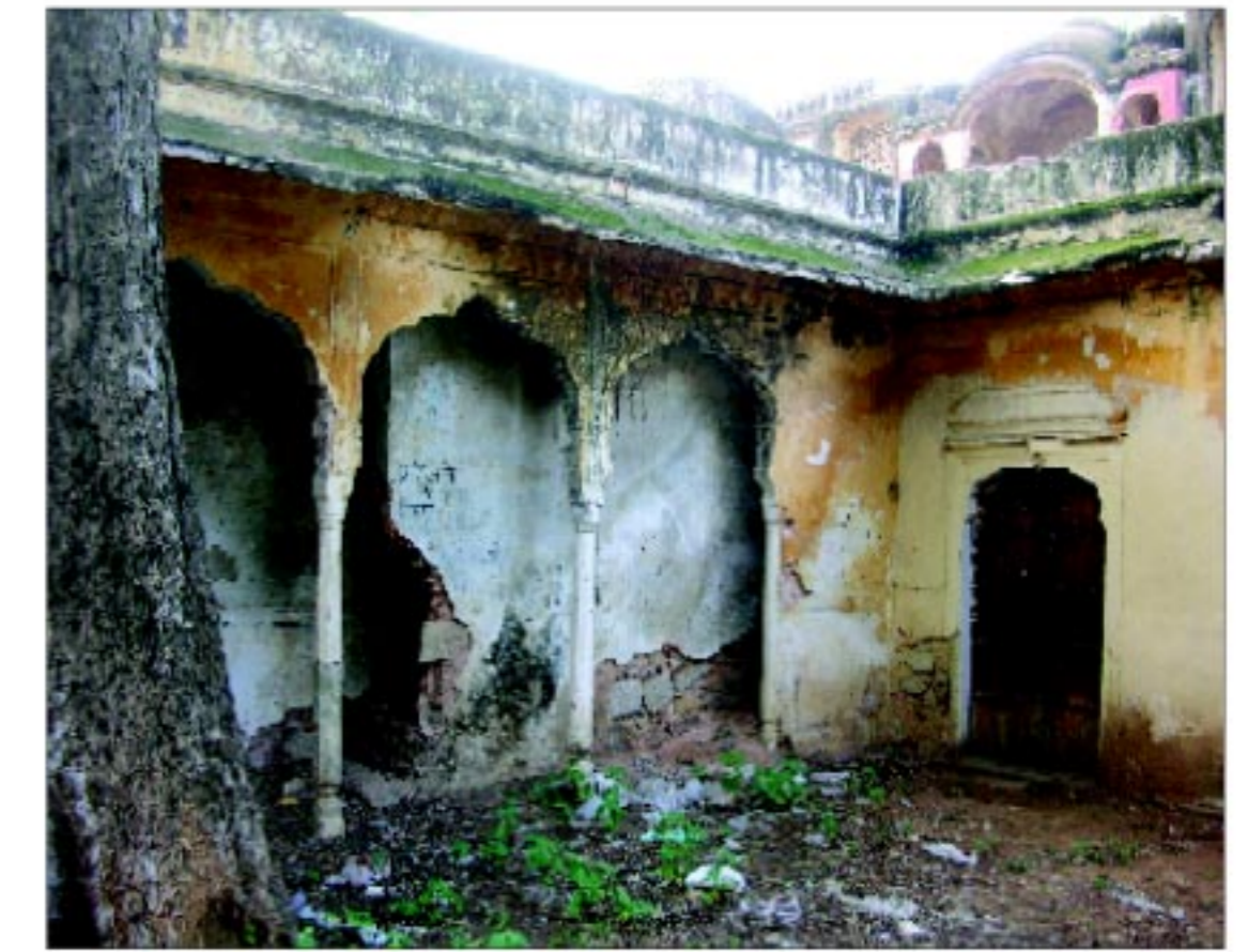
26. PLASTER PEEL OFF, WALL DAMAGED
