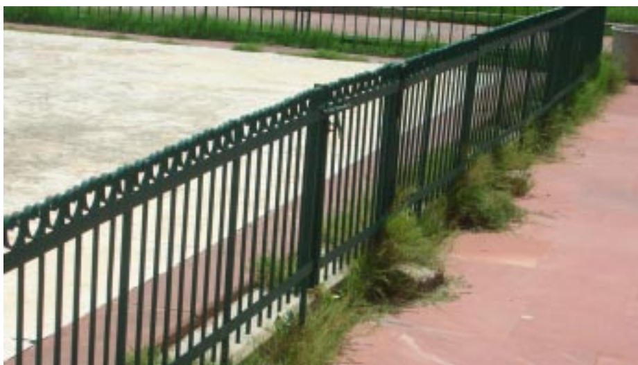
a. The railing and pathways all constitute the total ambience of the complex and are at the moment badly made and not maintained.
