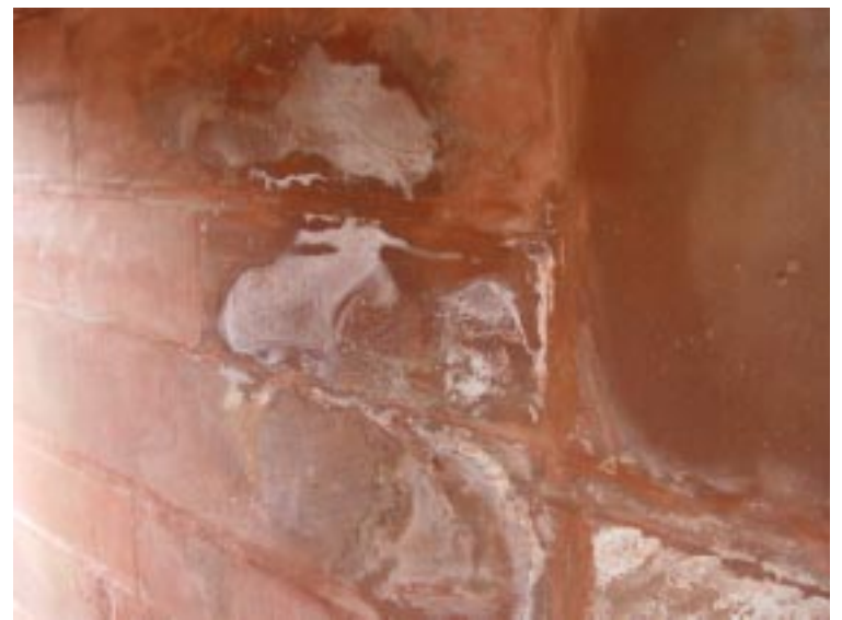
f. Efflorescence on the stone surfaces
