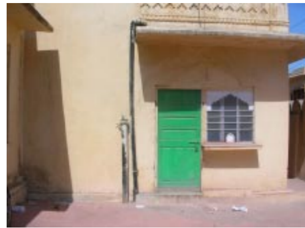
2. EXPOSED DRAINAGE PIPES
