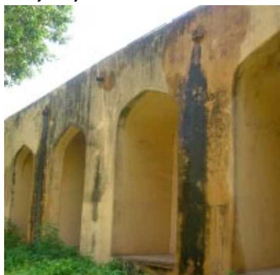
f. Algae formation due to water run off
