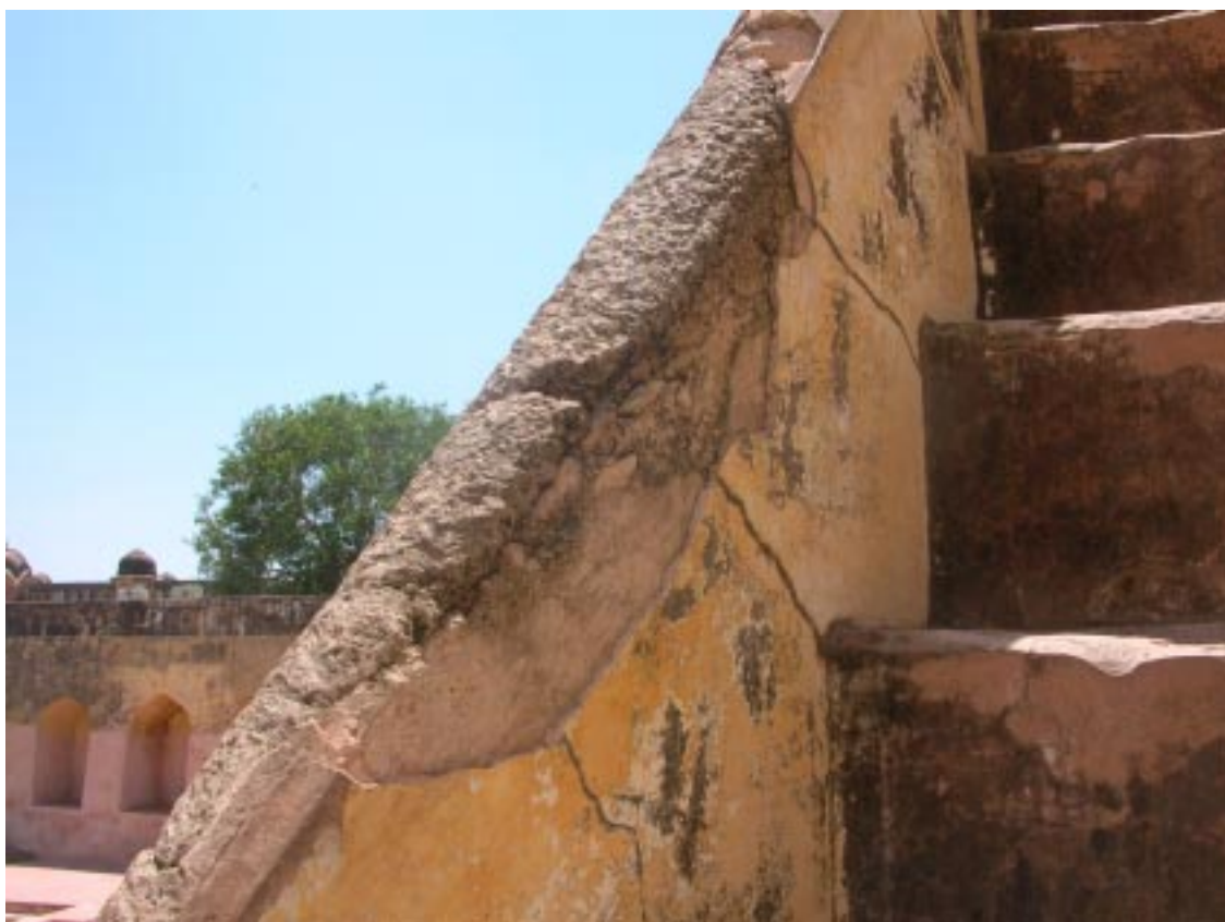
b. The surface plaster of the parapet has worn away exposing the stone
