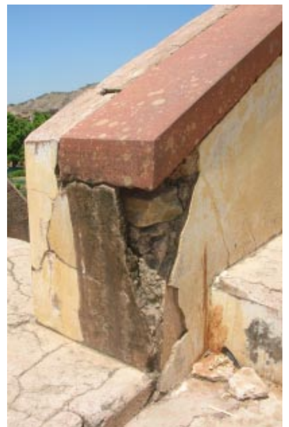
d. Deterioration of the parapet
