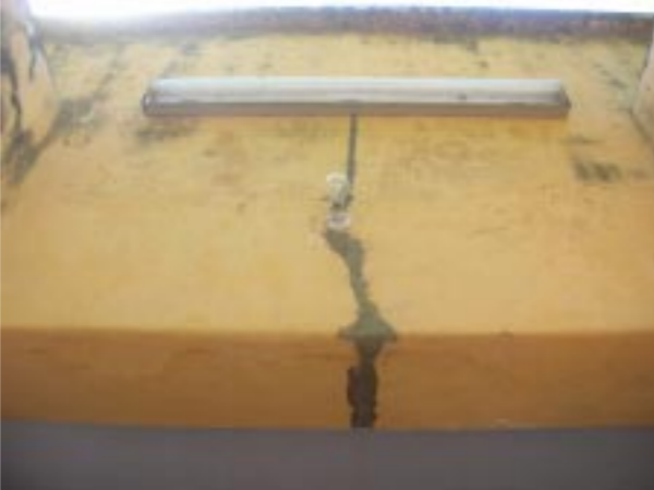
3. WALL CRACK AND REPLASTERING EXPOSED
