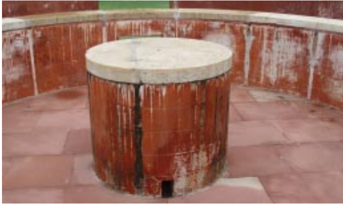
a. Lack of proper rainwater drainage causes damage to the markings.
