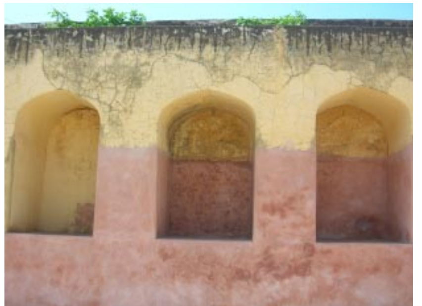
d. Replastering has not been matched with the earlier plaster
