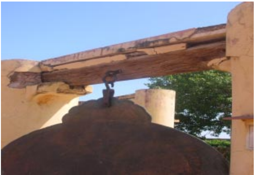
b. Structural damages like cracking of the load bearing timber beams in Yantra Raj
