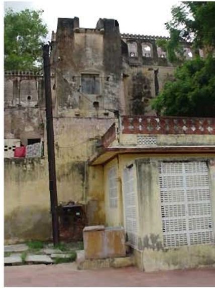
View of toilet block and exposed electrical meter box
