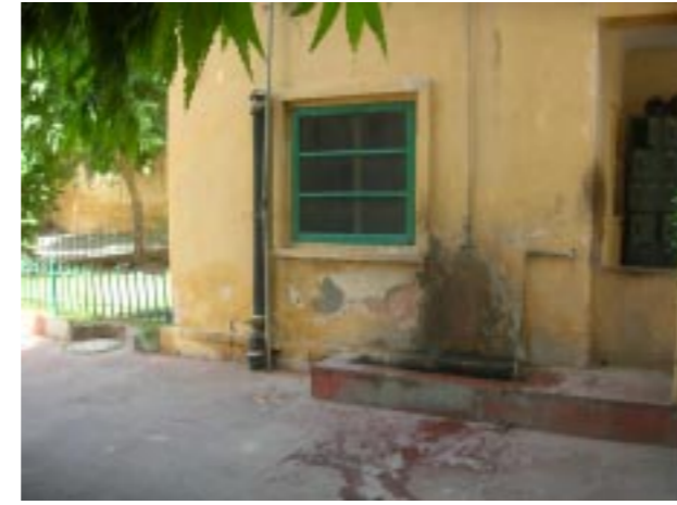
5. PLASTER PEEL OFF DUE TO WATER
