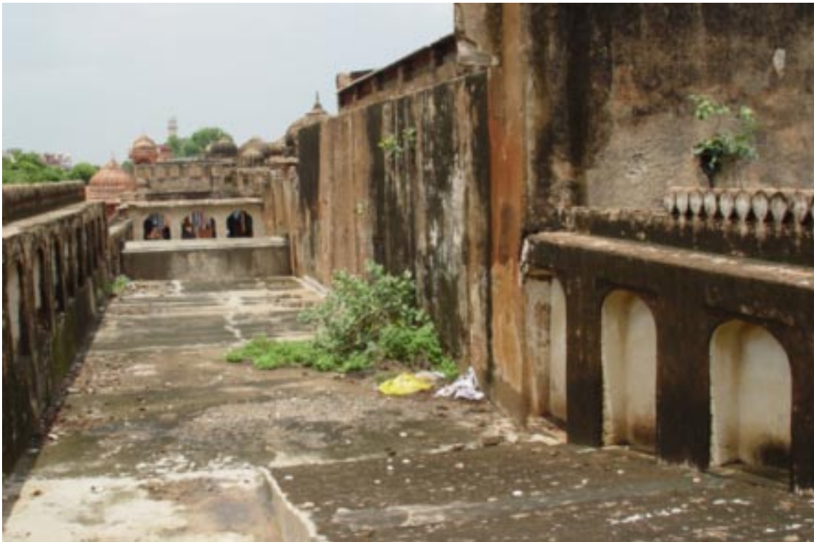
d. Presently the terraces of the buildings are in disuse and are easily accessible. They can, thus, be easily brought into use.
