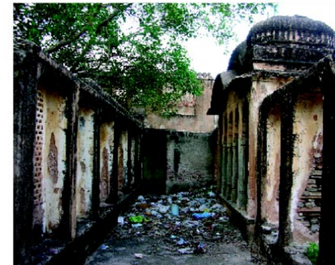
27. GARBAGE COLLECTION, PLASTER PEEL OFF
