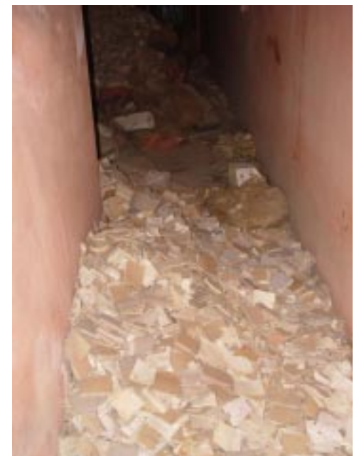
f. Dumping in closed rooms and corridors
