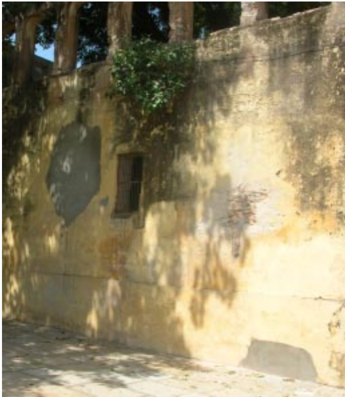
b. Uneven plaster patches.
