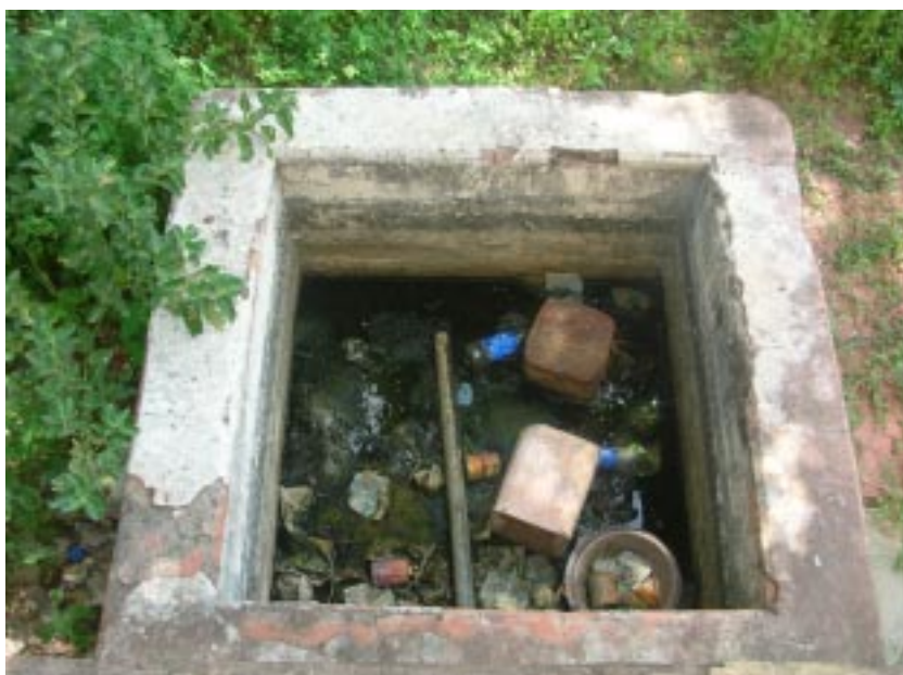
d. Garbage dumped in water sumps.
