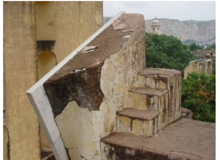
c. The chipping away and cracking of the plaster will eventually lead to damage of the yantra as the support becomes weak.
