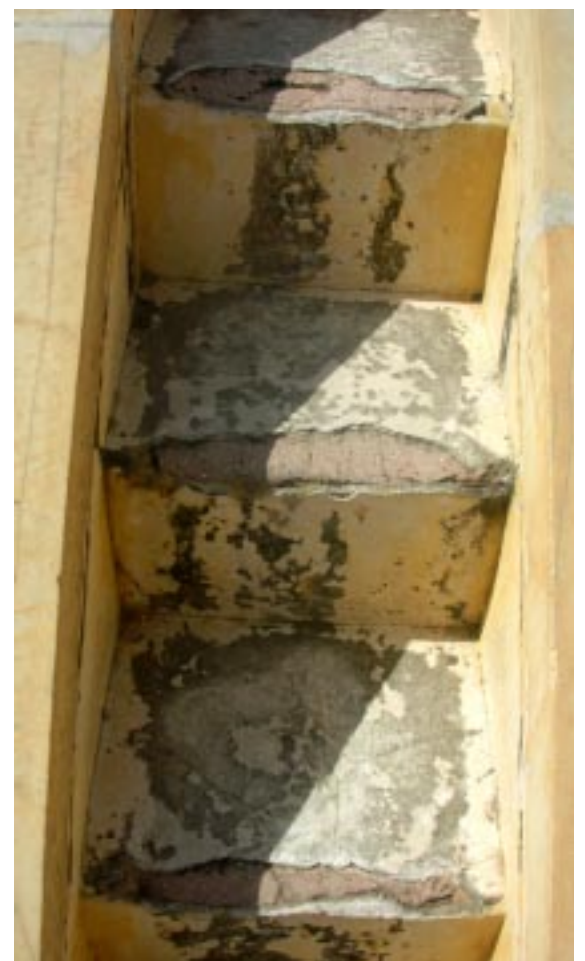
e. Wear and tear of steps
