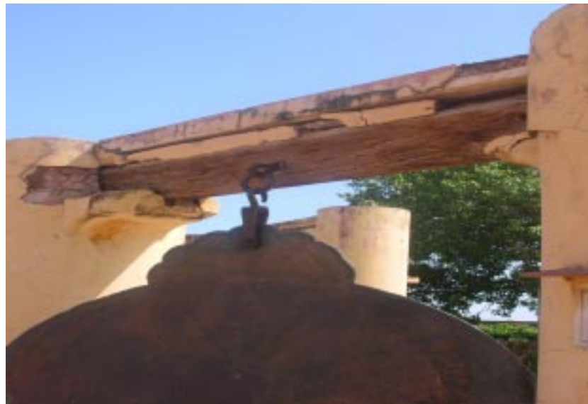
b. Structural damages like cracking of the load bearing timber beams in Yantra Raj
