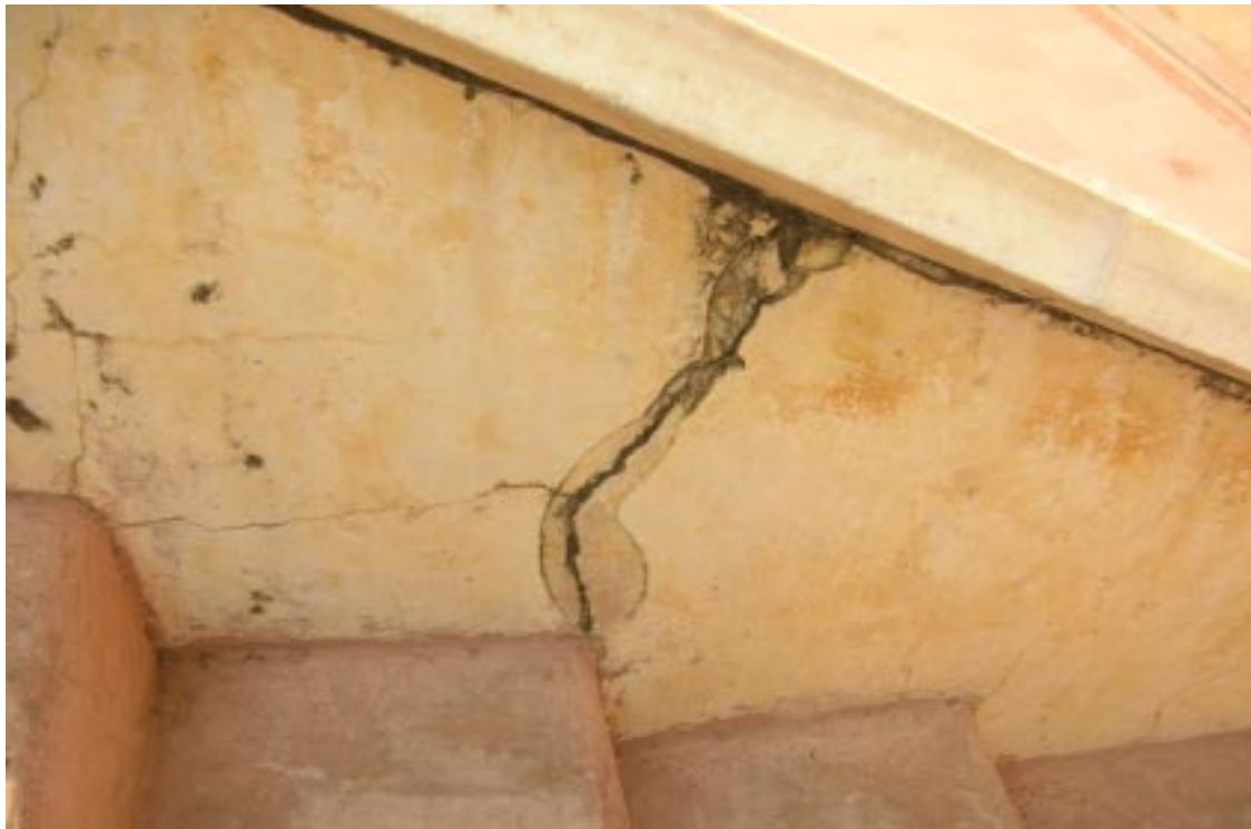
a. The parapet of the stair has cracked considerable. The parapet will most likely collapse if not repaired urgently
