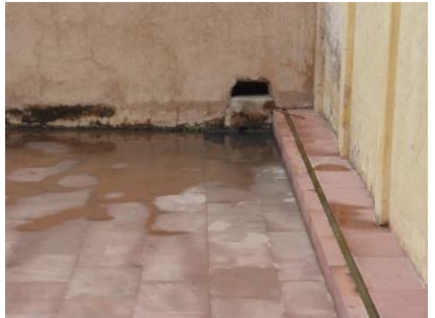
b. Ponding and improper water drainage systems causing water seepage.
