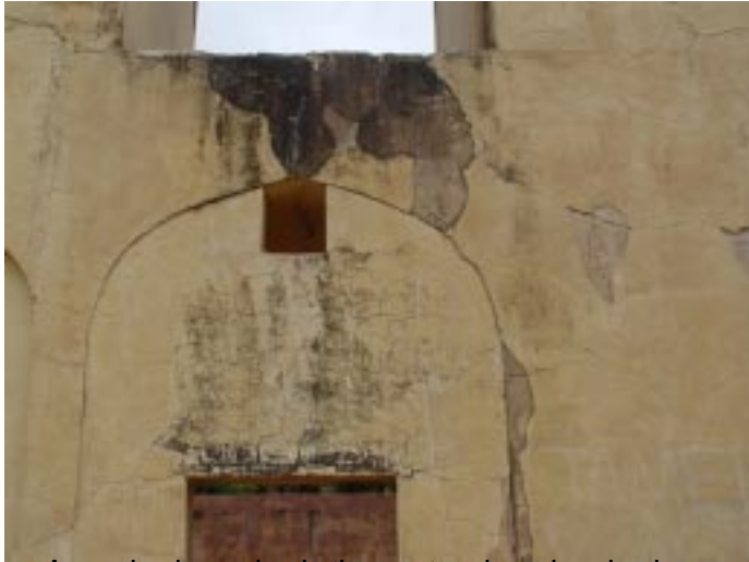
a. An arched opening in the yantra closed and a doorway made to access the portion behind.
