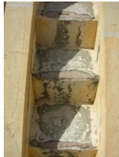
f. Wear and tear of steps
