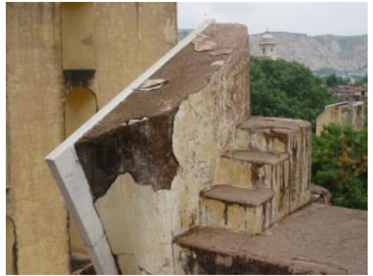
d. The chipping away and cracking of the plaster will eventually lead to damage of the yantra as the support becomes weak.
