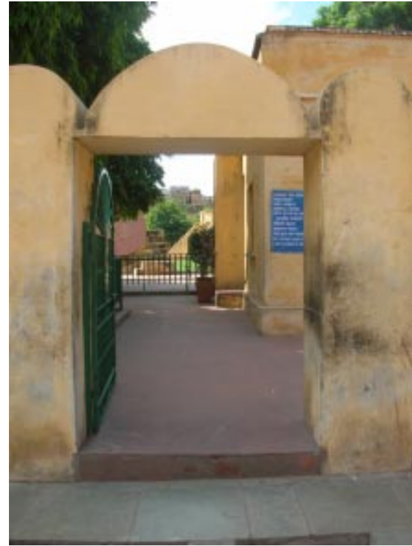
1. INAPPROPRIATE ENTRANCE GATE
