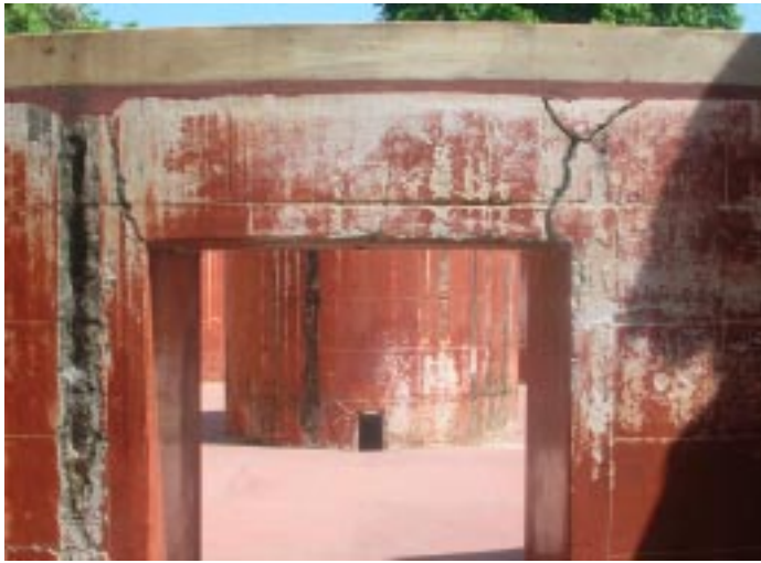
a. The lintels in the Digansha Yantra are cracking and need attention
