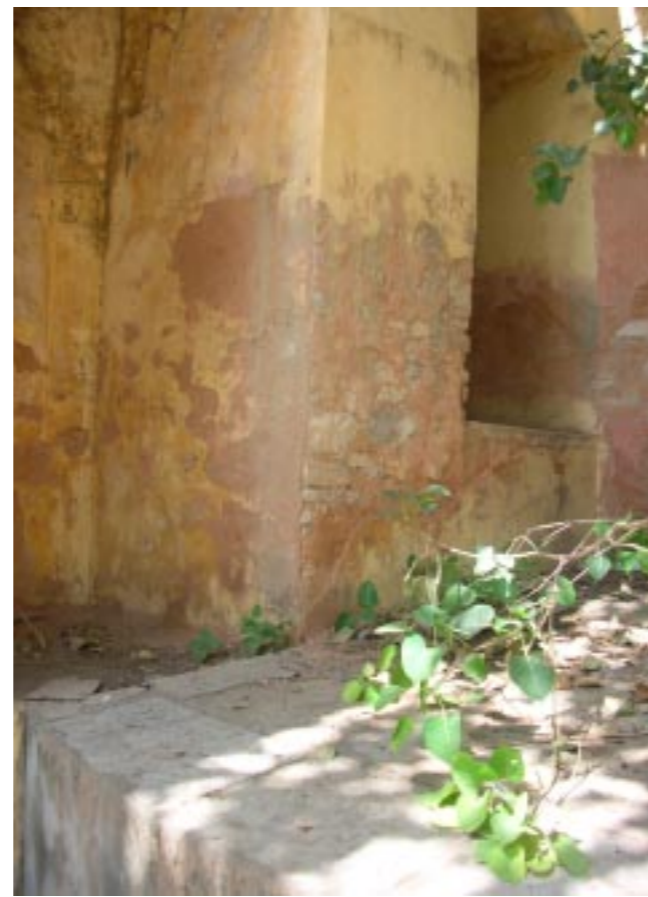
9. PLASTER PEEL OFF
