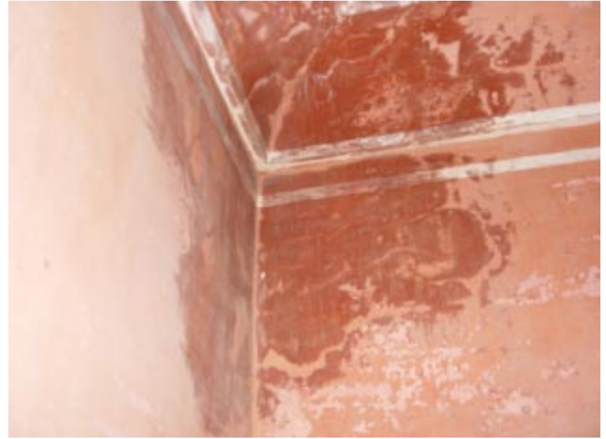
c. Dampness from water percolation will eventually weaken the structures leading to structural failure.
