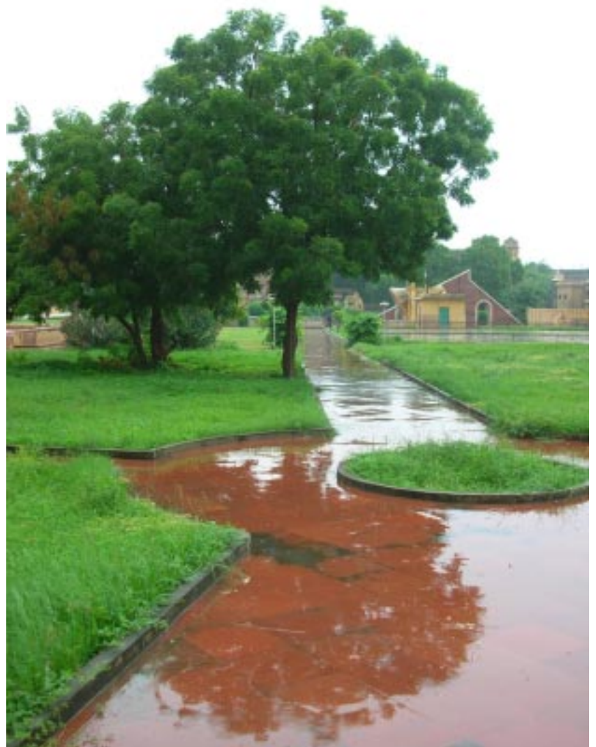
d. Ponding in the pathways will eventually damage them
