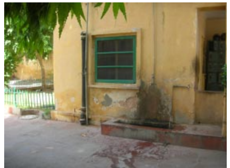
d. Washing area right in front of the entrance. It is also not properly made leaving lot of dampness and wet area.
