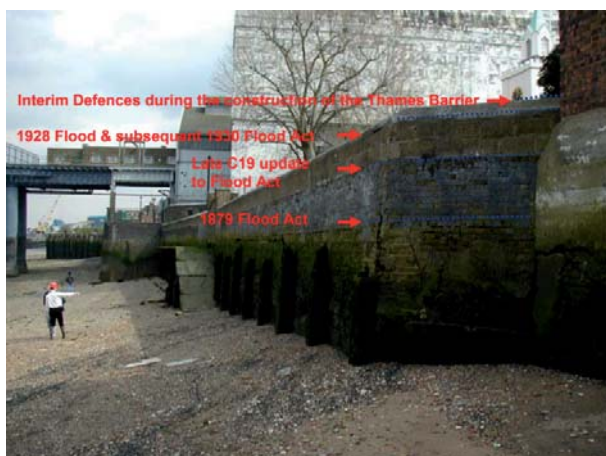
Figure 20: A traditional response to floods can lead to progressive unplanned adaptations, as seen here in the Thames a series of flood events lead to the need to raise and re-raise the flood walls
