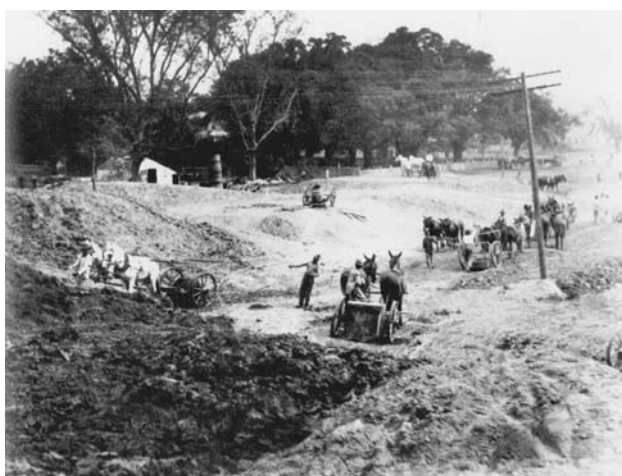
Figure 11: Material is delivered to an early levee construction on the Mississippi River (circa 1860–1925)
