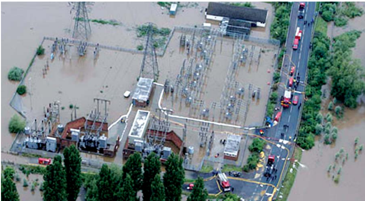
Figure 55: Castlemead power distribution station is inundated in July 2007, UK
