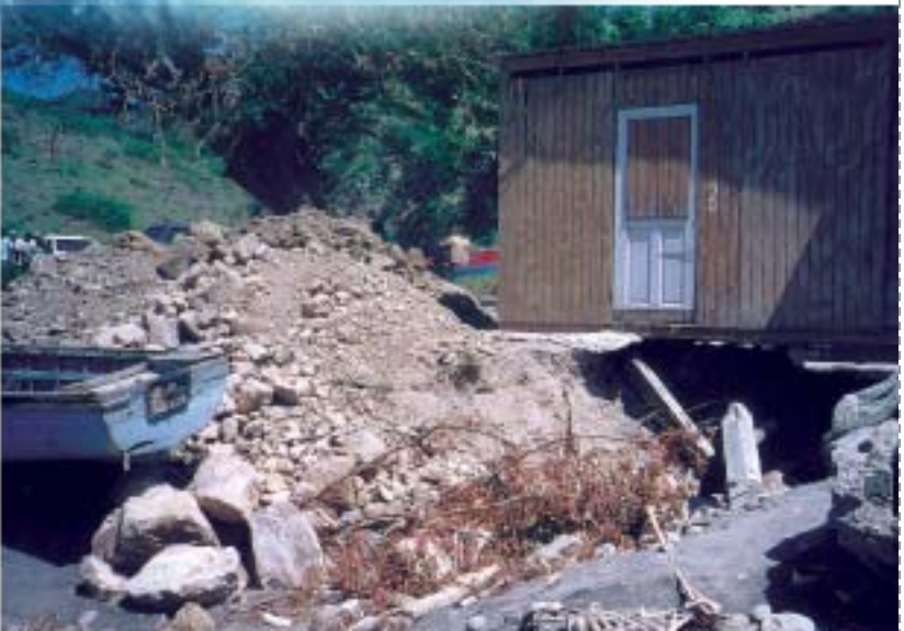
The foundations of this house at Carr's Bay were washed out during Hurricane Georges, 1998
