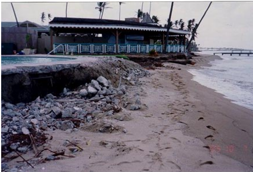
Pinney's Beach, October, 1995. Hurricane Luis eroded the beach and the land behind the beach undermining the foundations of the restaurant and the swimming pool. The implementation of adequate setback provisions would have prevented much of this damage.
