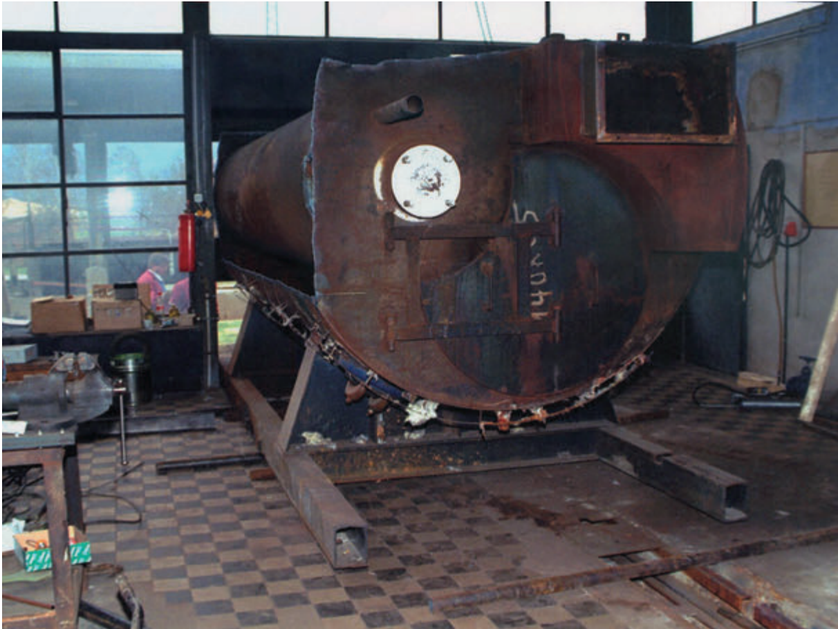
Fig. 76: Engine house, extension of the oil burner system (1994)
