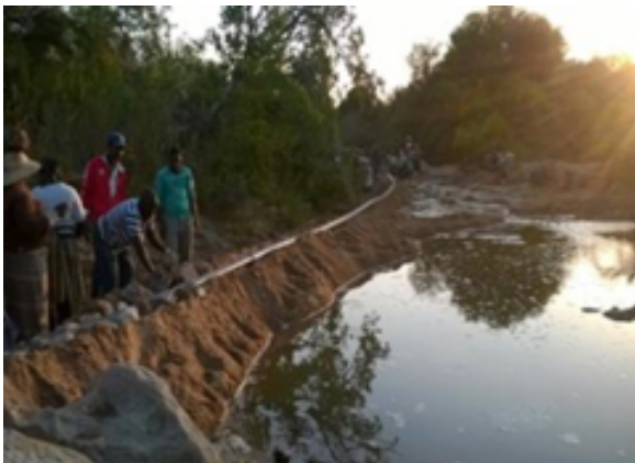
Putting the infiltration gallery in place (Swaziland) Photo: Department of Water Affairs (2014).
