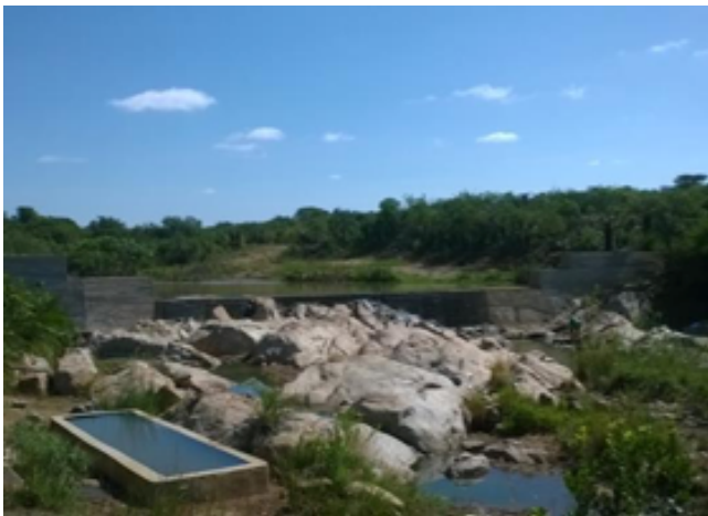
A sand dam with a properly built cattle trough downstream (Swaziland) Photo: Department of Water Affairs (2015).
