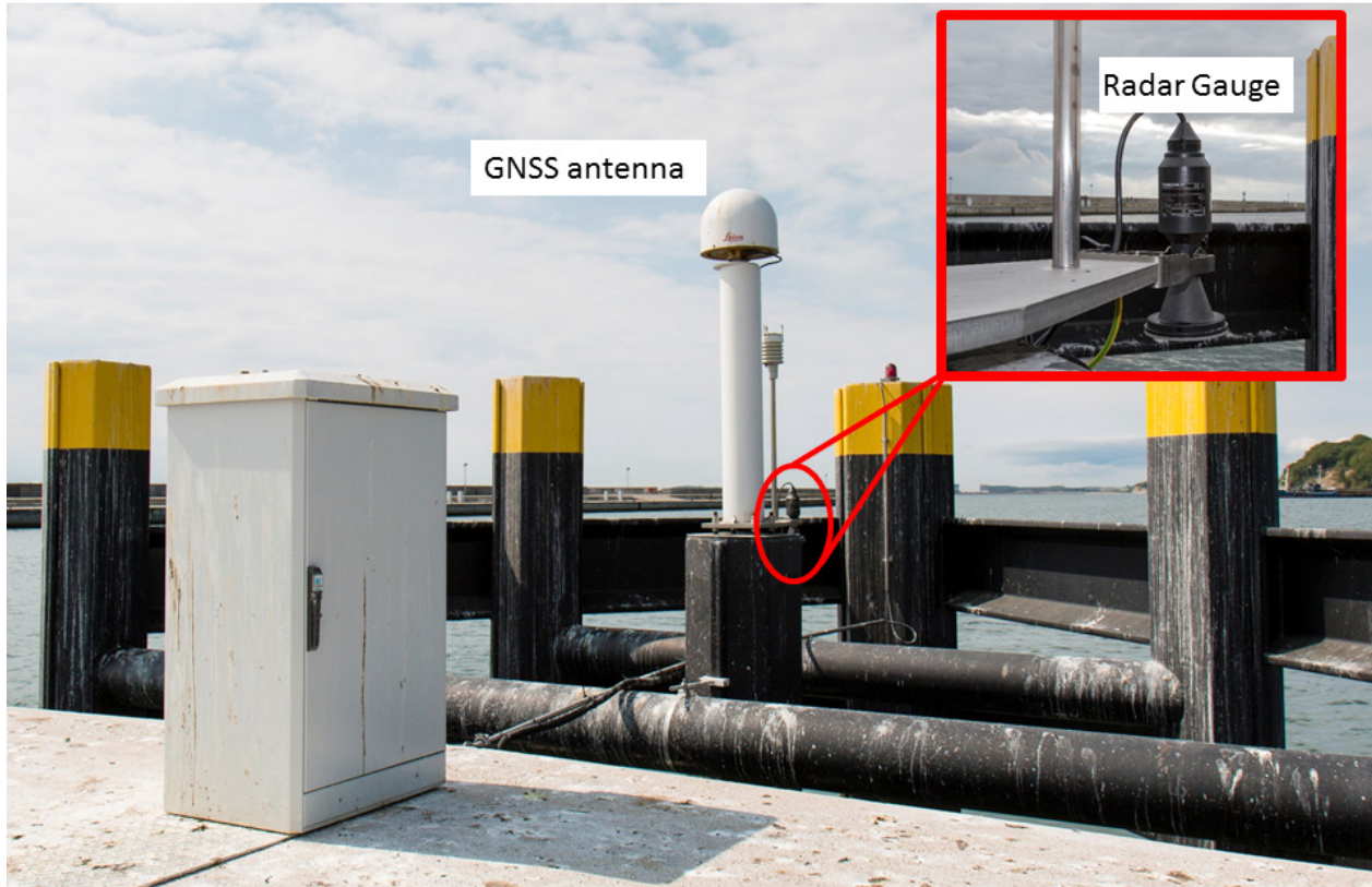
Figure 12 New GNSS reference station in Sassnitz (GREF station SAS2) with GNSS antenna on top of the antenna pillar, control unit, weather measurement unit and Radar Gauge (in operation since April 2016).
