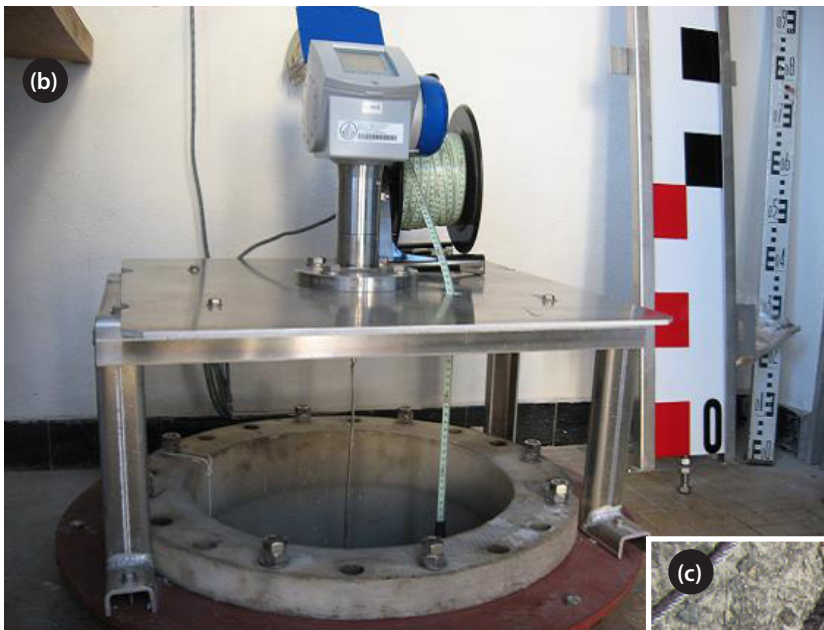
(b) A GWR sensor installed in an existing stilling well at Sète, France. (Photograph SHOM).
