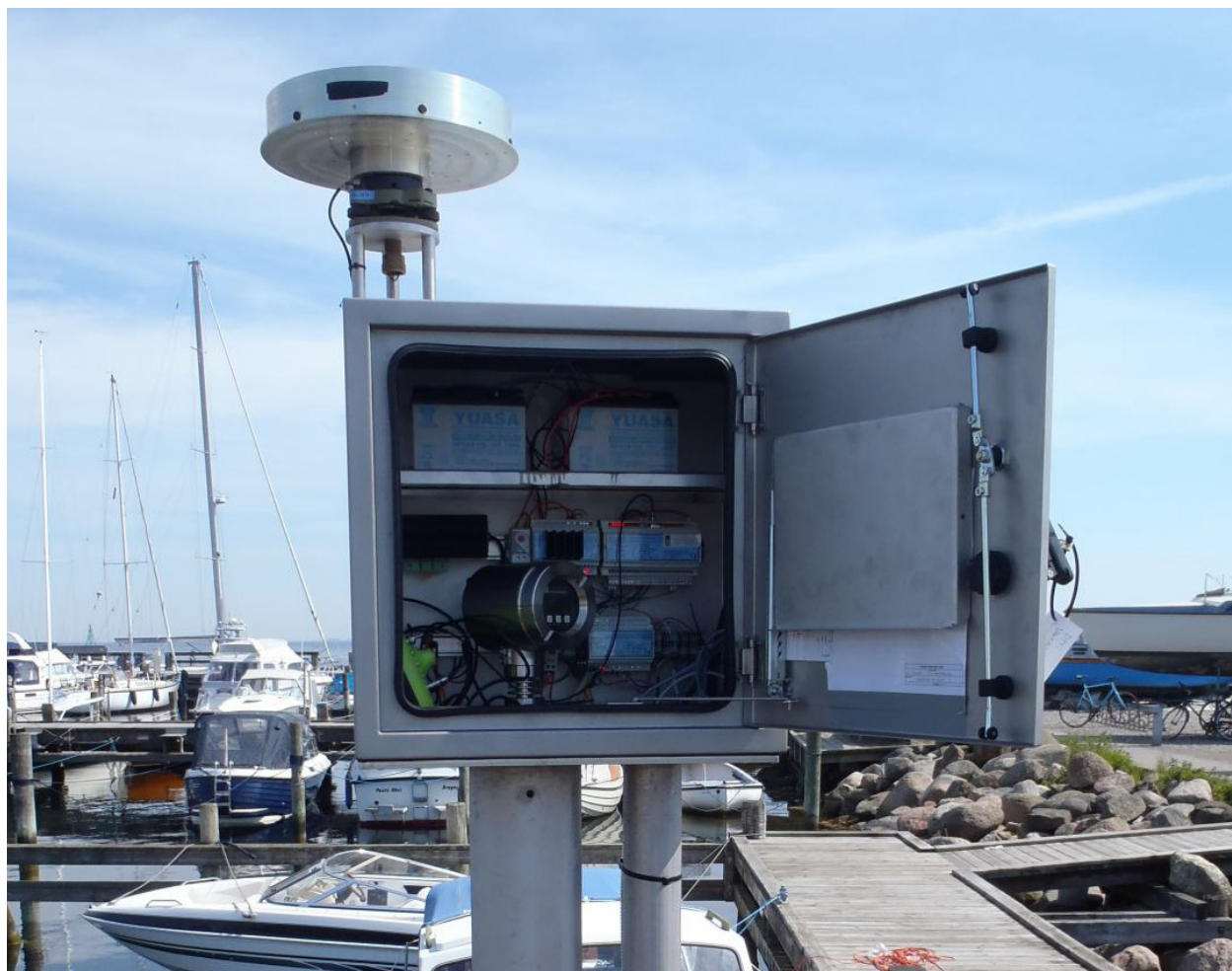
Figure 4.6 An installation at Dragør, Denmark. On the left can be seen an Endress+Hauser radar gauge mounted on top of a stainless steel tube (approximately 17 cm diameter) that functions as a stilling well and waveguide. This tube has an end cap with a 30 mm diameter inlet. Inside the tube is a filter to prevent biological intrusions. At the top of the tube are 4 holes with filters to prevent condensation on the radar antenna. On the right is a stainless steel tube containing pressure sensor cables. (Photograph Danish Meteorological Institute).
