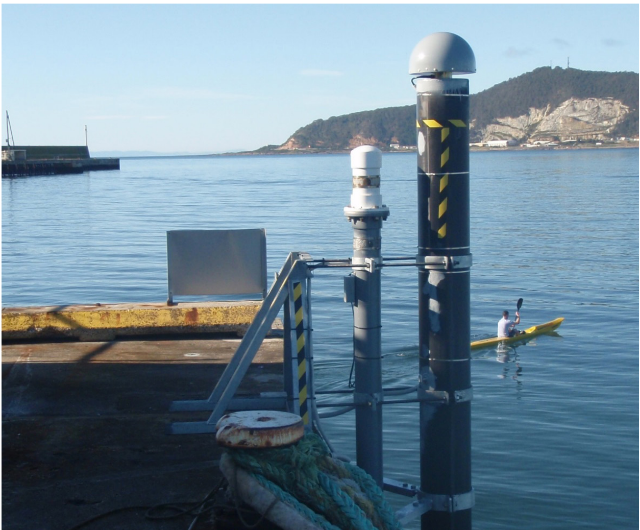
Figure 6.4 An acoustic tide gauge at Burnie in northern Tasmania, Australia, and, to its right, a special pillar with a GNSS antenna on top. Photograph courtesy of Geoscience Australia. From Pugh and Woodworth (2014).
