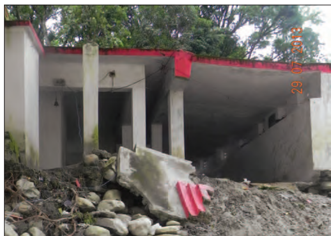
Figure 5: Damage to Lata Baba Temple due to flash floods in Sumadi, Rudraprayag
