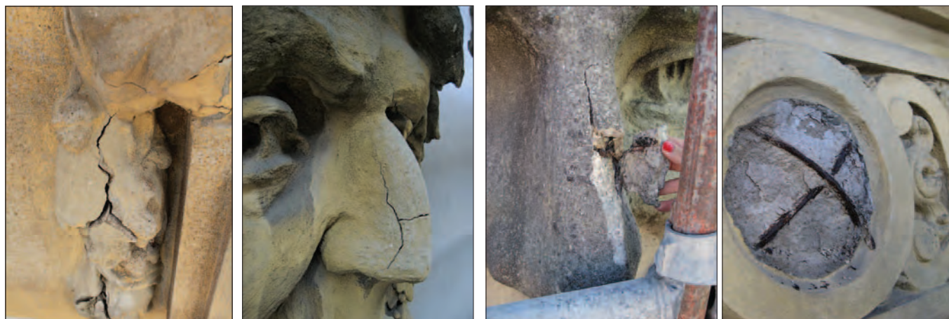
Figure 1 – Examples of reinforced concrete decorative elements and sculptures exhibiting some level of material degradation.
