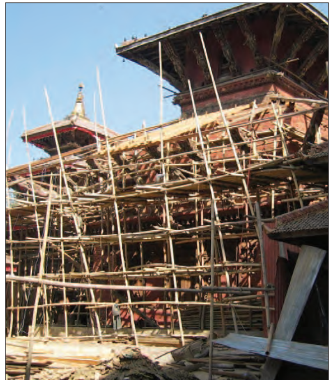
Figure 8: A temple under restoration: a typical process of restoration/reconstruction of timber and brick structures.
