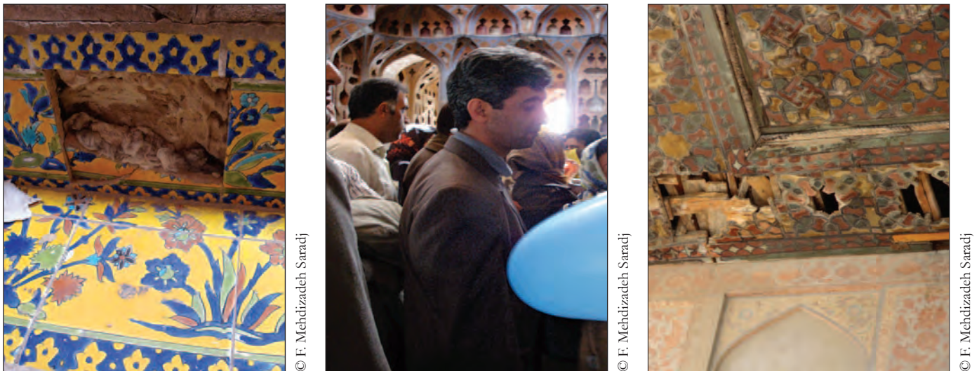
Figure 7: Threatening risks to Ali Qapu building owing to (a) The gradual attrition and the ignorance of stakeholders, (b) The unpredicted load on the structure by tourists during New Year vacation, (c) Rotting of the ceiling wooden parts in veranda due to the air pollution of the surrounding environments.
