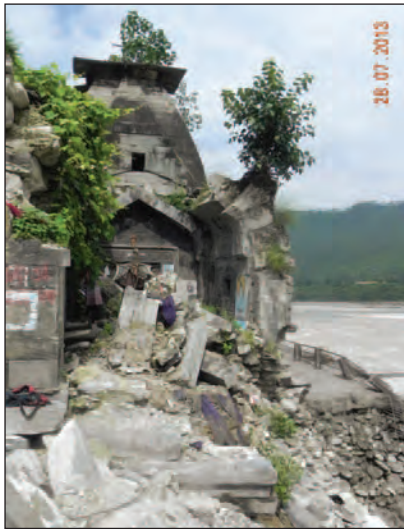
Figure 10: Image showing damage to Keshav Math in Srinagar
