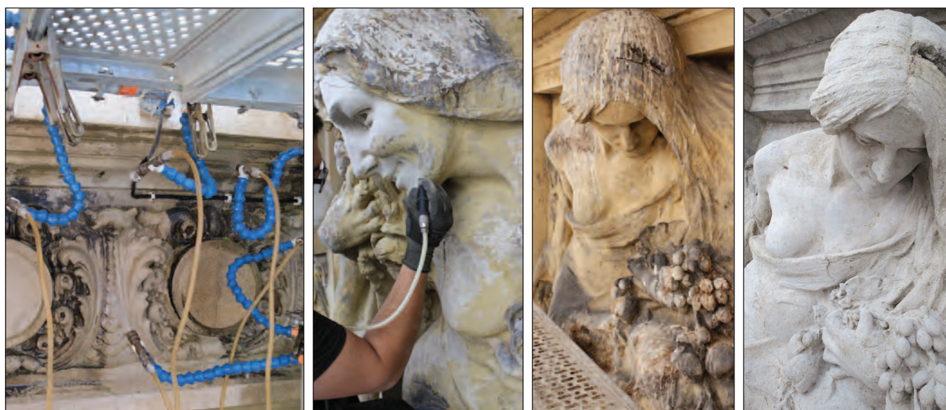
Figure 4 – Cleaning operation to remove limewash (left), cleaning operation by micro-abrasion (centre left), example of a decorative element before (centre right) and after (right) the cleaning operation.
