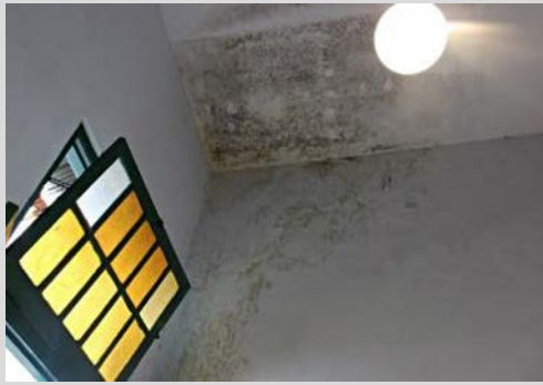
Figure 55: Ceiling and wall of Kedai Seni Jakarta (second floor) became humid and defective
