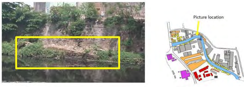
Figure V.24. Picture and location of the old canal wall from Dutch colonial period Source: Field Observation, 2015
