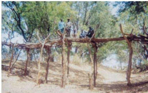
A wooden bridge built to access protected areas during the flooding season
