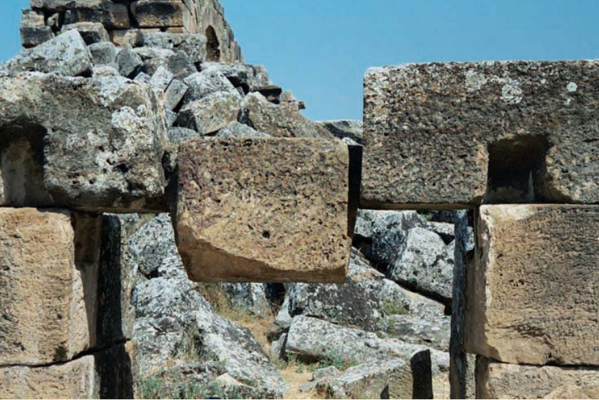
Typical earthquake-related structural damage pattern: a dropped keystone in a doorway near the Byzantine Gate in the Roman city of Hierapolis in southwest Turkey, near the modern town of Pamukkale, northeast of Denizli. © Manuel Sintubin
