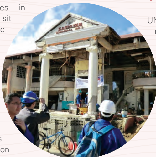
Post-disaster engineering field investigation of building damage. Bohol, Philippines © UNESCO/ S. Yasukawa
