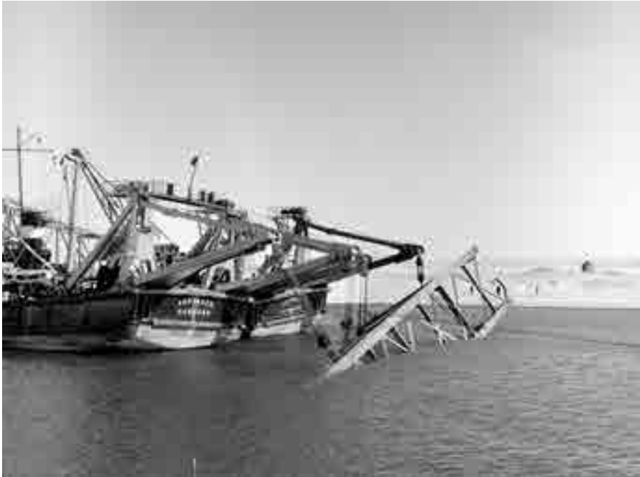
I-7.3 Clearing the Suez Canal; the UN salvage fleet lifts and removes the damaged eastern section of the al-Ferdan bridge
