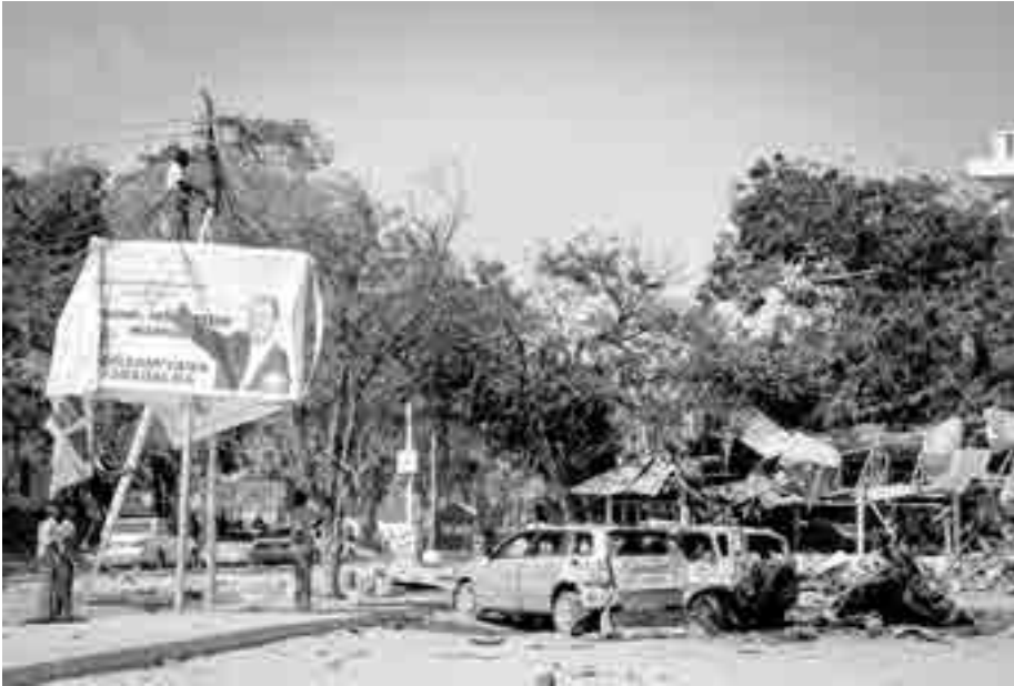
III-9.2 Repairs begin after a double suicide attack by the al-Qaeda-affiliated extremist group al-Shabaab killed 18 people and injured dozens more at a restaurant in Mogadishu, Somalia in September 2013
