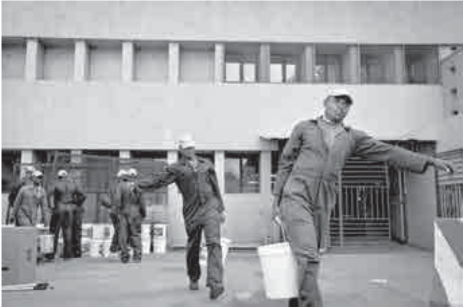
V-4.3 UN workers from Ghana renovating a school in Taliko, a marginalized neighbourhood of Bamako, Mali. The school had hosted several displaced families after deadly flash floods hit the Malian capital in the summer of 2013
