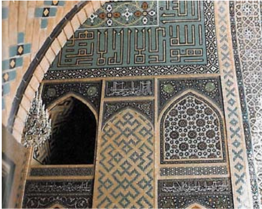
Fig. 38. Mashhad. View of the western aiwān of the Friday mosque. (Photo: Courtesy of H. R. Zohoorian.)
