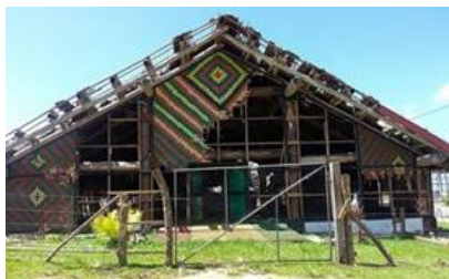
Cultural Heritage damage at Vanuatu
