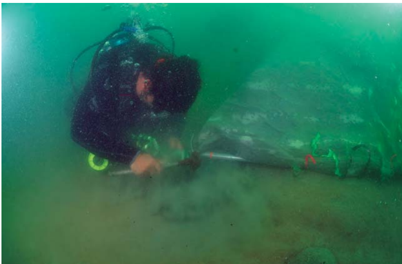
Artificial seagrass is being installed on the seabed. This self-made grass is temporary covered with a sheet to prevent the fronds from floating up while installing it. © UAD, Thailand
