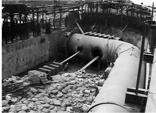
Fig. 47 Visiting gallery installed in the protection shell cavities (III)
