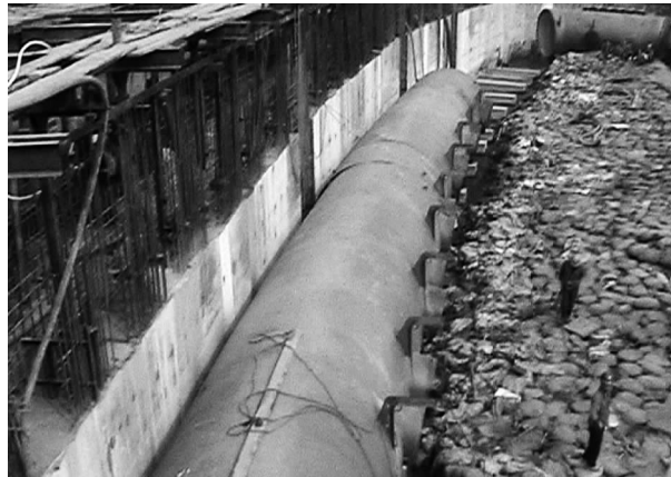
Fig. 45 Visiting gallery installed in the protection shell cavity (I)
