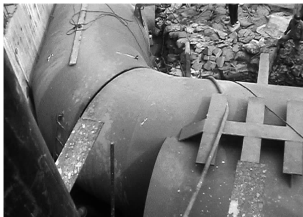
Fig. 46 Visiting gallery installed in the protection shell cavity (II)
