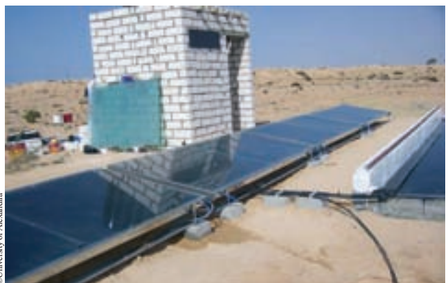
Two days later, the system is nearly ready for use. More panels will be added to increase the capacity and a wall will later be constructed to shield the material from sandstorms and intruders
