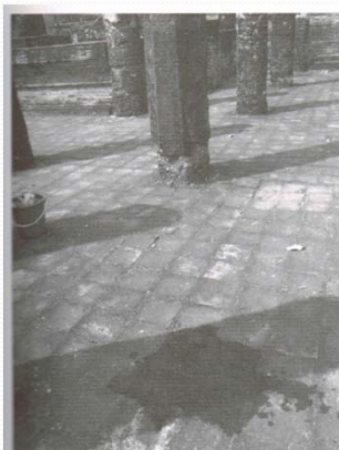
25) Part of brick floor at Wat Sa Si just after application of the new type biocide
