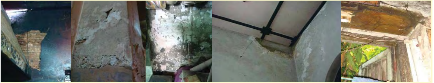
Interior deterioration due to humidity and negligence
