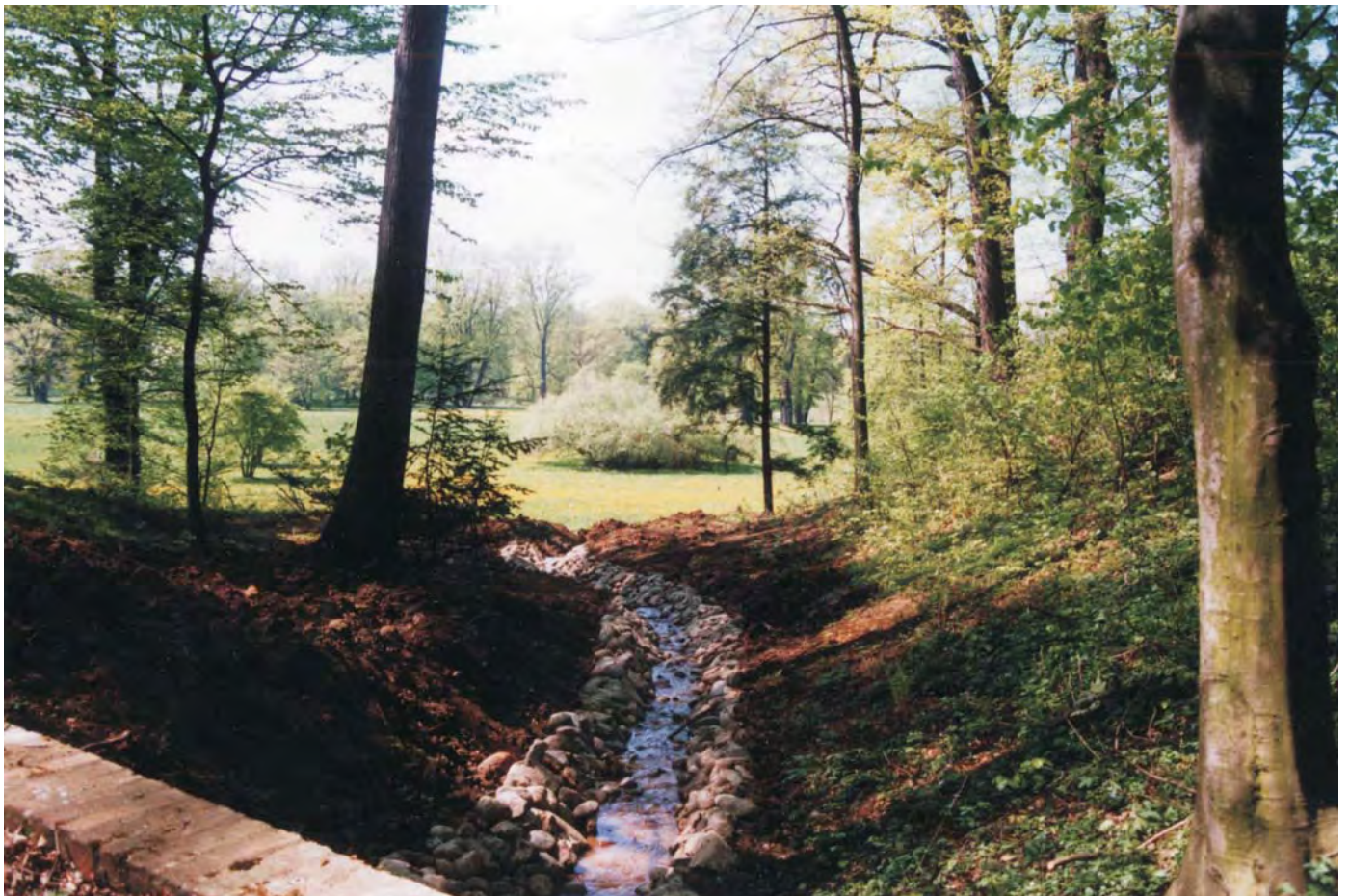
40. Part of the drainage ditch in the Park on Terraces (Polish side)
