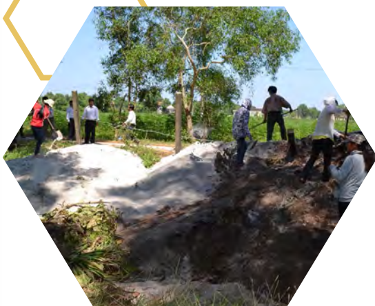
The deep holes in the schoolyard were filled in as part of the implementation of the plan for the 2013-2014 academic year, with the active support of parents and community members.
