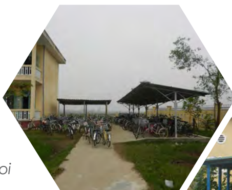
The school parking lot is covered by iron sheets that pose a hazard during storms.
