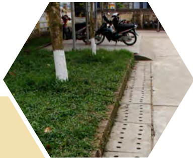
25m of drainage system was built in front of the school with the support of the Parents Association and contributions from community members.
