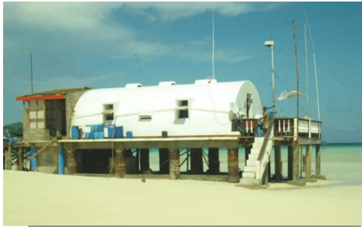
Photo of the expansion of the ranger station, where a water cistern and new septic tank was constructed under the floor. Fresh water has been a major limitation. The cistern is now in use. Finishing touches will be completed by early March.
