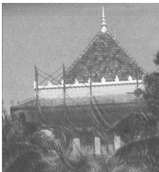
The Hotel Renakse is now barred to visitors, wrapped in netting and slated for demolition. TRACEY SHELTON
