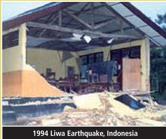
Figure 2.11: Out-of-plane failure of brick masonry wall
