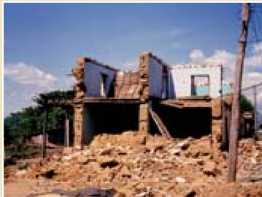
b) Damaged Tapial
