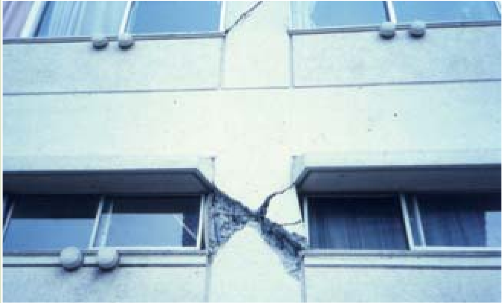
Figure 8.4: Diagonal shear cracks of a short column (1995 Kobe Earthquake, Japan)
