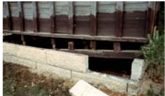
Damaged in 1978 Miyagi-ken-oki Earthquake, Japan
