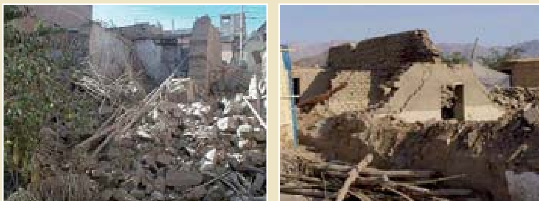
Figure 7.5: Damaged adobe (2007 Pisco Earthquake, Peru)
