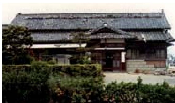
Damaged wooden house in 1978 Miyagi-kenoki Earthquake, Japan
