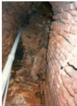
Collapsed portion of Santo Domingo tunnel.
