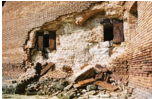
Failure at scarp wall.
