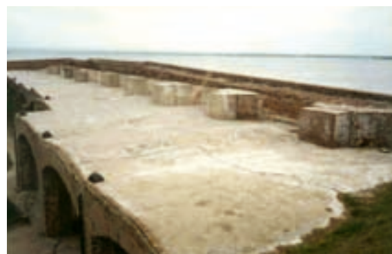
Left flank casemates at Fort Sumter before treatment.
