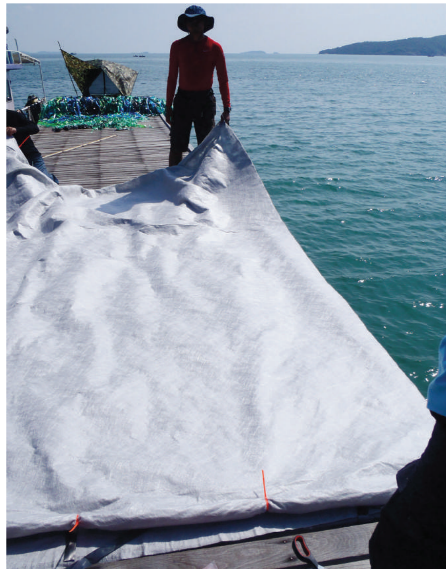
Geotextile is being fixed to a heavy iron pole before taken into the water, which reduces the buoyancy. © UAD
