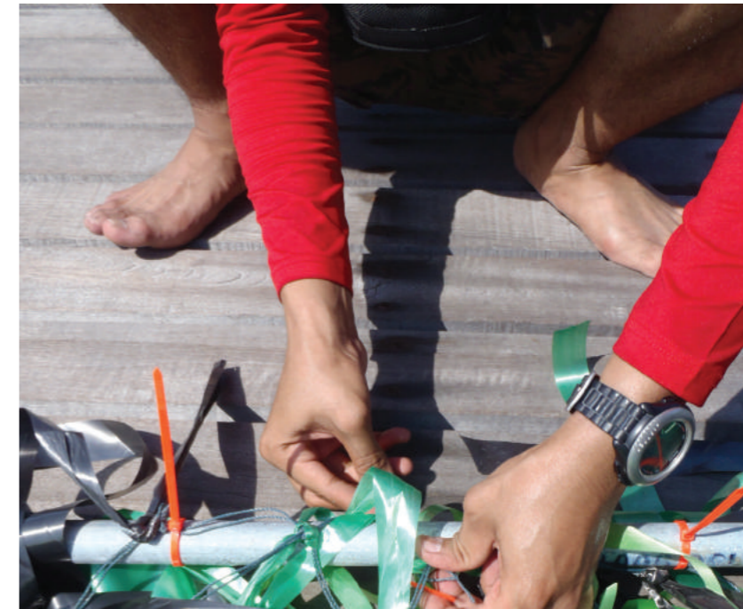
Like debris nets and geotextile, it is easier to install the artificial seagrass on the seabed when it is fixed to a heavy iron pole. © UAD
