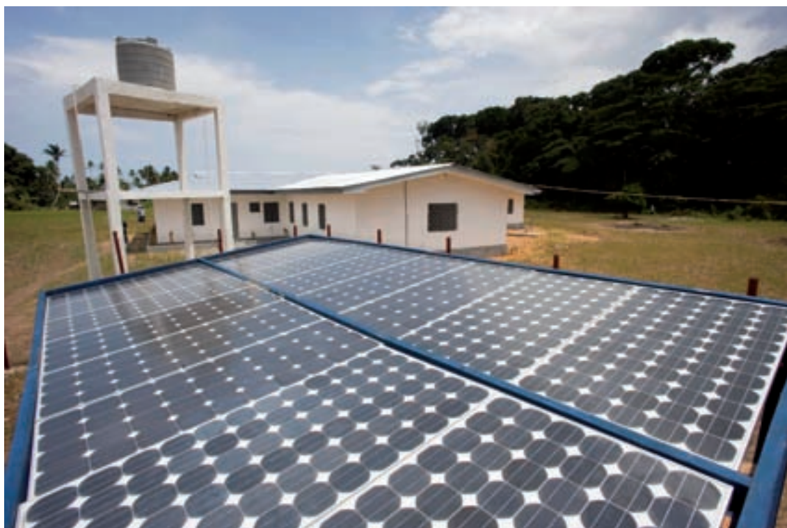
Solar power panels generate energy for a renovated local administrative building, erected by the Government of Liberia. Credit: UN Photo/Christopher Herwig.
