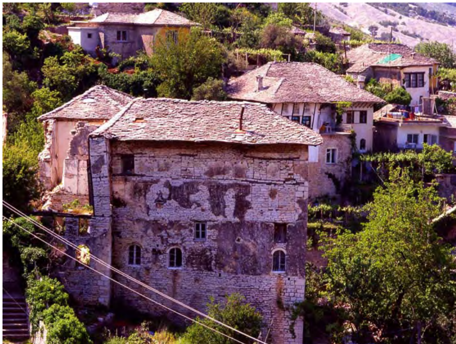
Fig. 18 – The Kabilati house largely in ruins
