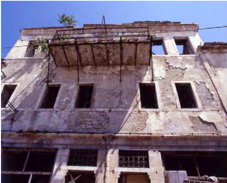
Fig. 33 – The upper storeys in the bazaar are often derelict
