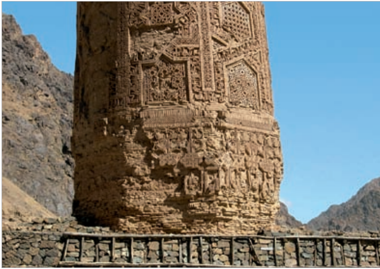
Fig. 2 | Repair work on the damaged gabions around the Minaret of Jam (2003). PHOTO: © UNESCO/F. LANGLOIS
