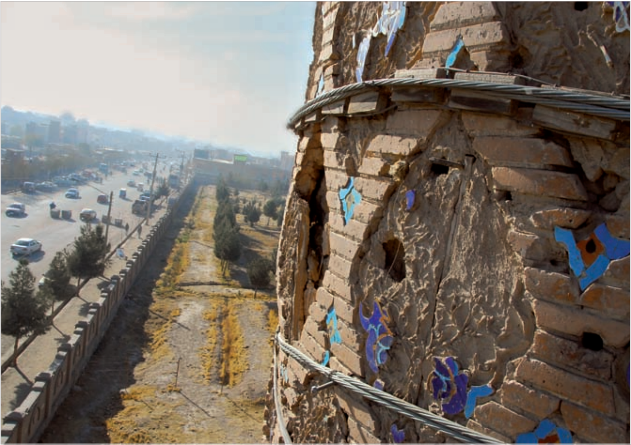
Fig.19 | Inspection of the stays supporting the Fifth Minaret (2010). PHOTO: © UNESCO/ C. MARGOTTINI
