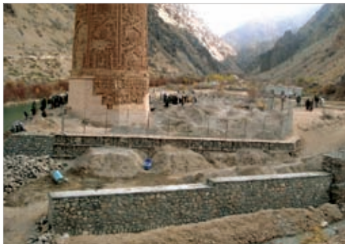
Fig. 9 | Overview of construction work during the River Defense Project (2007). PHOTO: © UNESCO/T. STEVENS
