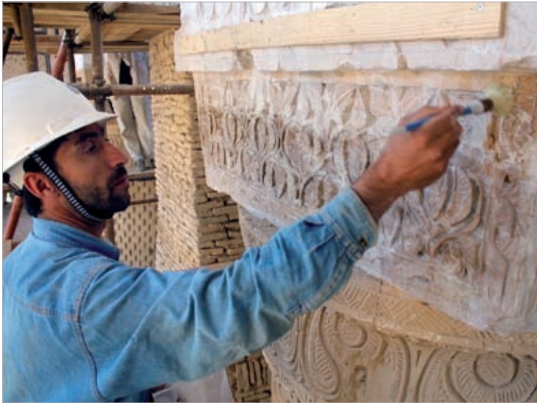
Fig. 2 | Before structural consolidation work could commence, the exquisite stucco decoration adorning the surfaces of the building had to be stabilized and protected.
