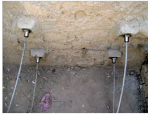
Fig. 20 | LEFT: Corroded stays of the Fifth Minaret (2010). PHOTO: © UNESCO/ A. LODIGIANI RIGHT: Replacement of the corroded stays of the Fifth Minaret (2012). PHOTO: © UNESCO/ K. KHAIRZADA
