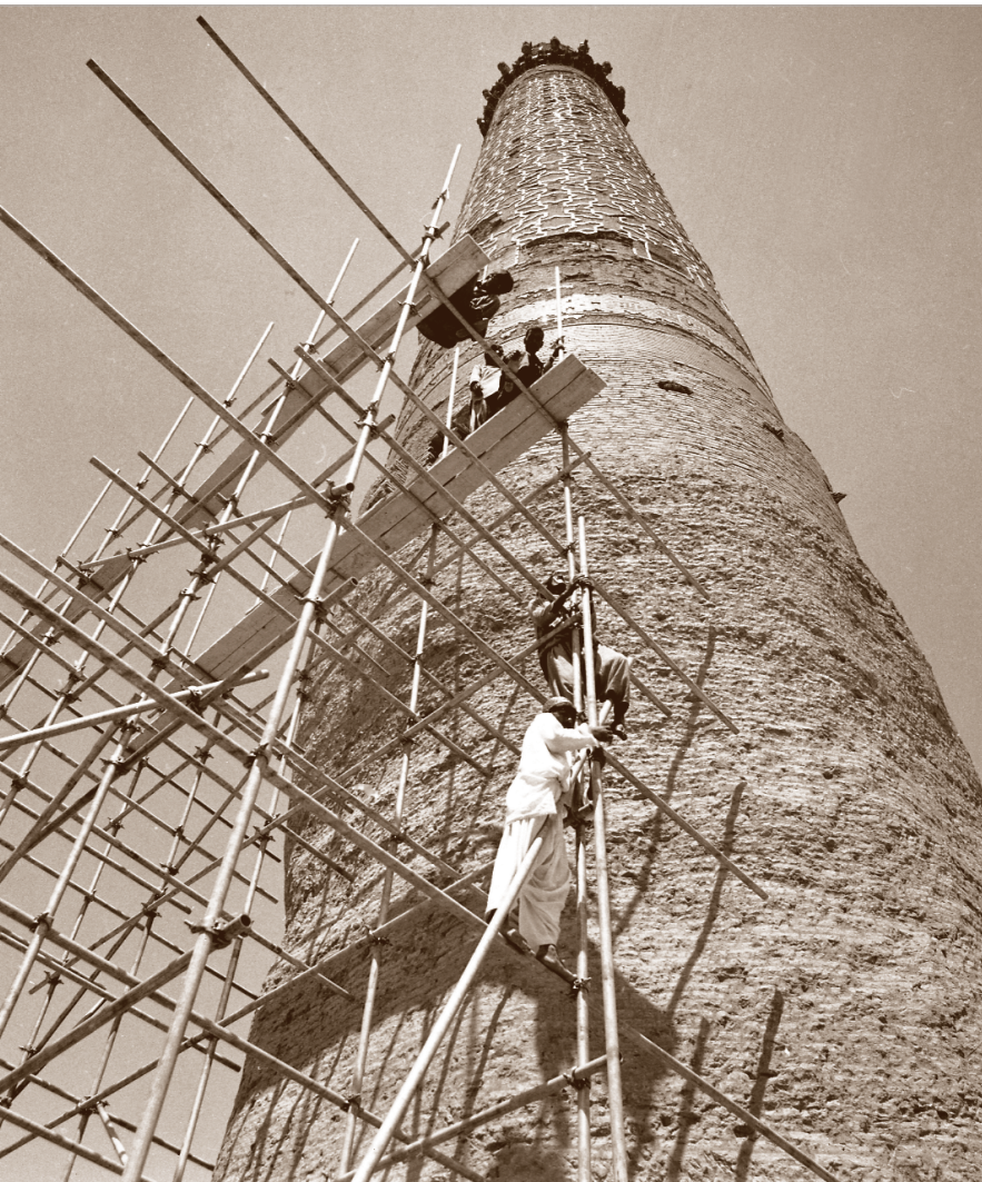
Fig.13 | Assembly of scaffolding to reach the entrance of the Minaret No.3 of the Husain Baiqara Madrasa, Herat (1977-79). PHOTO: ©A. BRUNO
