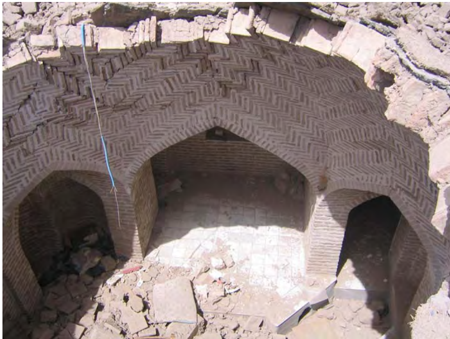
Fig.52. Seyed Abbas Bath after earthquake
