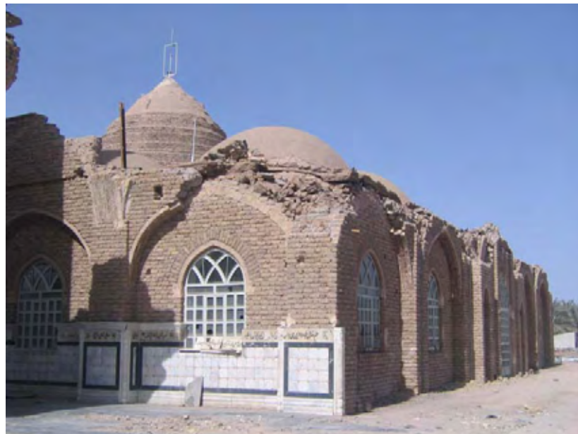
Fig.56. Emānzādeh Zeyd Mausoleum after the earthquake
