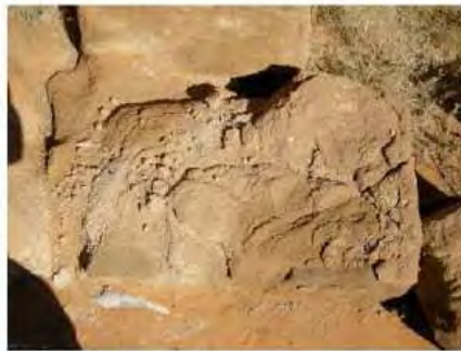
DSCN4132.JPG, Naqaa, Amun Temple, Degradation of Stone/ Masonry Elements
