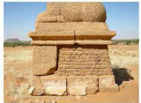
DSCN4079.JPG, Naqaa, Amun Temple, Exposure and Deterioration of Ancient Plasters
