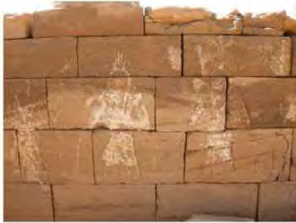
DSCN4084.JPG, Naqaa, Amun Temple, Exposure and Deterioration of Ancient Plasters, Degradation of Stone/Masonry Elements
