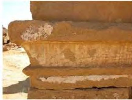
DSCN4073.JPG, Naqaa, Amun Temple, Exposure and Deterioration of Ancient Plasters
