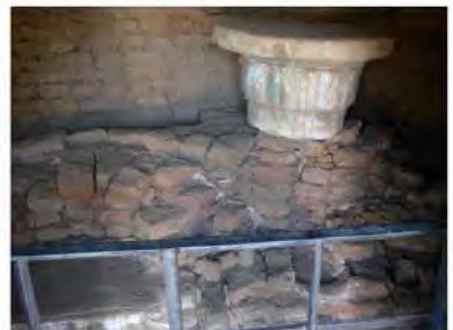
DSC06267.JPG, Degradation of Stone/Masonry Elements, Exposure and Deterioration of Ancient Plasters, Royal City
