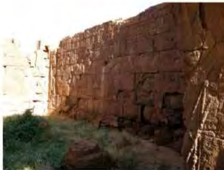
DSCN4025.JPG, Lion Temple B300 - Naqaa, Naqaa, Degradation of Stone/Masonry Elements, Inappropriate/Inexistent Site Drainage, Vegetation Damage
