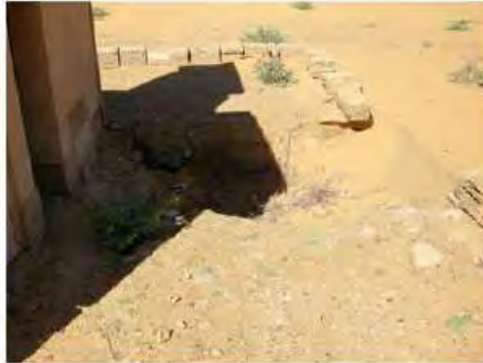
DSCN3834.JPG, Water Damage, Southern Cemetery
