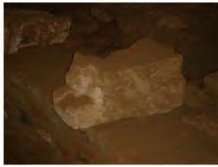
DSC06256.JPG, Degradation of Stone/Masonry Elements, Inappropriate/Inexistent Site Drainage, Royal City
