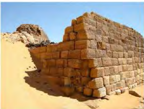
DSCN3753.JPG, Structural Deterioration of Pyramids, Northern Cemetery
