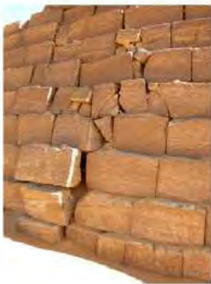
DSCN3741.JPG, Structural Deterioration of Pyramids, Northern Cemetery
