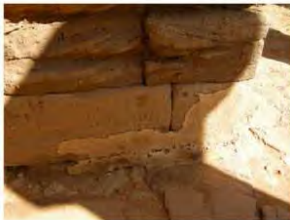
DSCN4098.JPG, Naqaa, Amun Temple, Exposure and Deterioration of Ancient Plasters, Degradation of Stone/Masonry Elements
