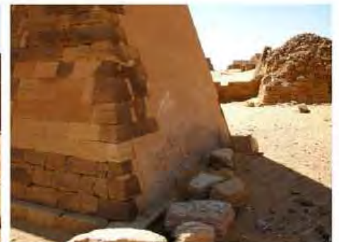
DSCN3779.JPG, Failure of Past Repair Work, Henkel Restoration, Salt Crystallization, Northern Cemetery
