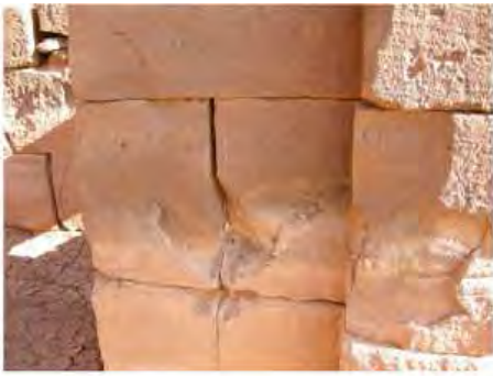
DSCN4009.JPG, The Kiosk - Naqaa, Naqaa, Degradation of Stone/ Masonry Elements, Inappropriate/Inexistent Site Drainage
