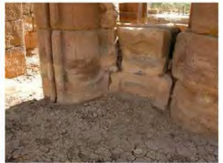
DSCN4004.JPG, The Kiosk - Naqaa, Naqaa, Degradation of Stone/ Masonry Elements, Inappropriate/Inexistent Site Drainage
