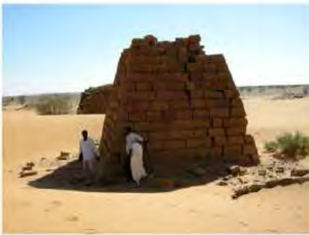
DSCN3860.JPG, Structural Deterioration of Pyramids, Southern Cemetery
