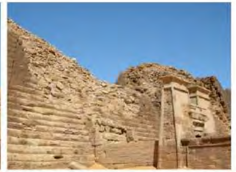
DSCN3770.JPG, Structural Deterioration of Pyramids, Northern Cemetery
