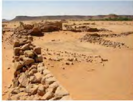
DSCN4174.JPG, Musawwarat - Great Enclosure, Structural Instability of Walls/Collapse of Archaeological Features, Structural Instability of Walls/Collapse of Archaeological Features
