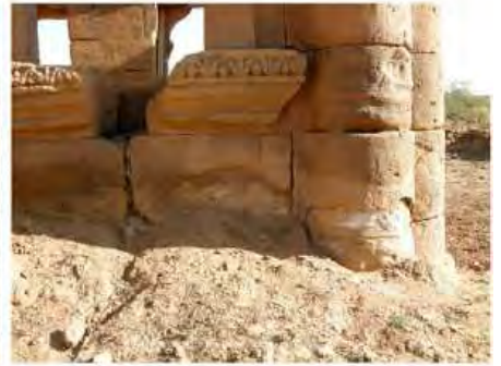
DSCN4001.JPG, The Kiosk - Naqaa, Naqaa, Degradation of Stone/ Masonry Elements, Inappropriate/Inexistent Site Drainage
