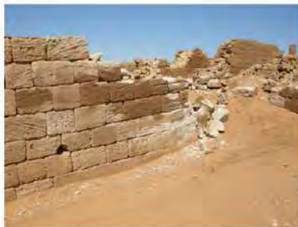
DSCN4171.JPG, Musawwarat - Great Enclosure, Degradation of Stone/Masonry Elements, Structural Instability of Walls/Collapse of Archaeological Features, Structural Instability of Walls/Collapse of Archaeological Features, Salt Crystallization
