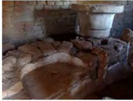
DSC06269.JPG, Inappropriate/Inexistent Site Drainage, Degradation of Stone/Masonry Elements, Exposure and Deterioration of Ancient Plasters, Royal City
