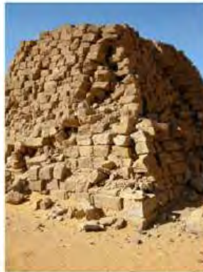
DSCN3862.JPG, Structural Deterioration of Pyramids, Southern Cemetery
