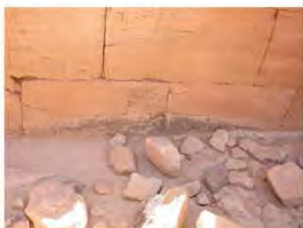
DSCN4145.JPG, Naqaa, Temple F, Inappropriate/Inexistent Site Drainage, Water Damage
