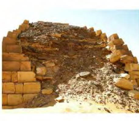
DSCN3742.JPG, Structural Deterioration of Pyramids, Northern Cemetery
