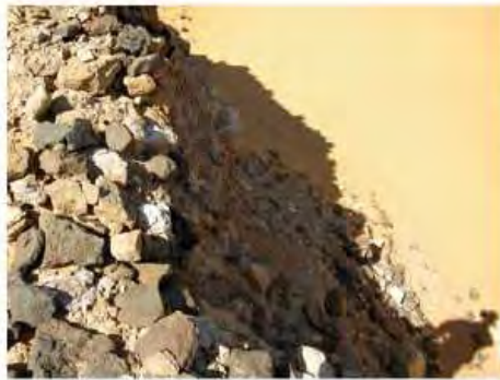
DSCN3733.JPG, Structural Deterioration of Pyramids, Northern Cemetery
