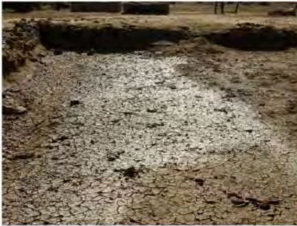
DSCN4013.JPG, The Kiosk - Naqaa, Naqaa, Inappropriate/Inexistent Site Drainage
