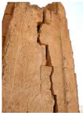
DSCN4152.JPG, Naqaa, Temple F, Structural Instability of Walls/Collapse of Archaeological Features, Exposure and Deterioration of Ancient Plasters, Structural Instability of Walls/Collapse of Archaeological Features
