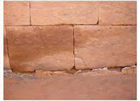
DSCN4129.JPG, Naqaa, Amun Temple, Exposure and Deterioration of Ancient Plasters, Inappropriate/Inexistent Site Drainage
