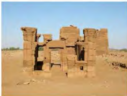
DSCN3995.JPG, The Kicek - Naqaa, Naqaa, Degradation of Stone/Masonry Elements, Inappropriate/Inexistent Site Drainage, Site Wide View
