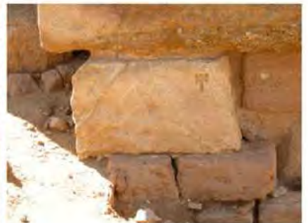
DSCN4121.JPG, Naqaa, Amun Temple, Exposure and Deterioration of Ancient Plasters, Degradation of Stone/Masonry Elements
