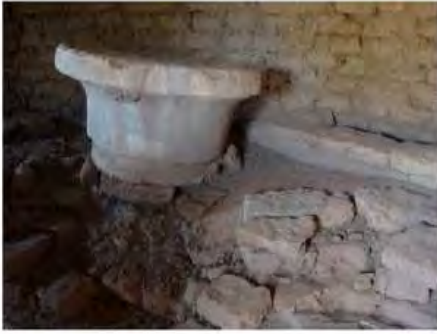
DSC06268.JPG, Exposure and Deterioration of Ancient Plasters, Degradation of Stone/Masonry Elements, Inappropriate/Inexistent Site Drainage, Royal City
