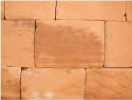
DSCN4176.JPG, Musawwarat - Great Enclosure, Degradation of Stone/Masonry Elements, Salt Crystallization
