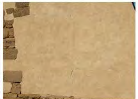
DSCN3829.JPG, Failure of Past Repair Work, Southern Cemetery
