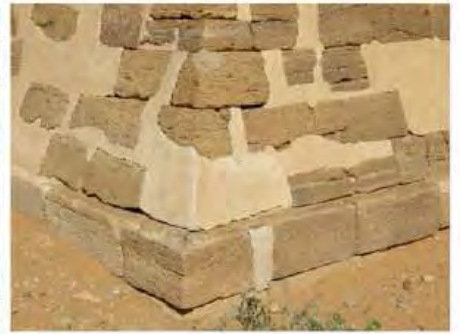
DSCN3832.JPG, Unsympathetic Repair Work/Interventions, Southern Cemetery
