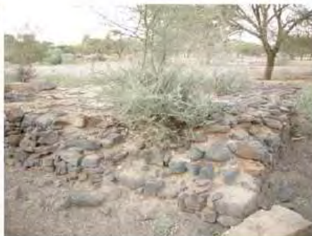
DSCN3939.JPG, Vegetation Damage, Structural Instability of Walls/Collapse of Archaeological Features, Royal City
