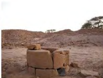
DSCN3963.JPG, Inappropriate Dumping of Excavation Spoils, Structural Instability of Walls/Collapse of Archaeological Features, Degradation of Stone/Masonry Elements, Inappropriate/Inexistent Site Drainage, Royal City
