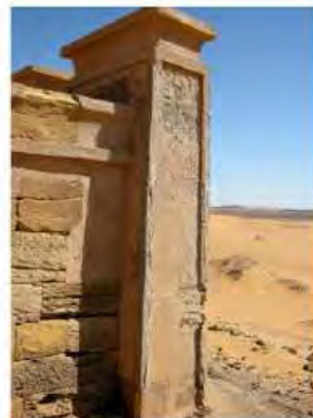
DSCN3718.JPG, Failure of Past Repair Work, Northern Cemetery
