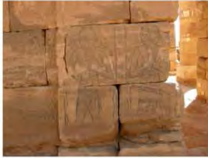
DSCN4096.JPG, Naqaa, Amun Temple, Degradation of Stone/Masonry Elements, Structural Instability of Walls/Collapse of Archaeological Features
