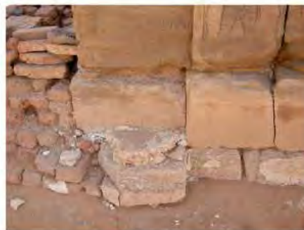
DSCN4094.JPG, Naqaa, Amun Temple, Degradation of Stone/Masonry Elements, Exposure and Deterioration of Ancient Plasters
