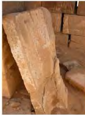
DSCN4086.JPG, Naqaa, Amun Temple, Exposure and Deterioration of Ancient Plasters, Structural Instability of Walls/Collapse of Archaeological Features
