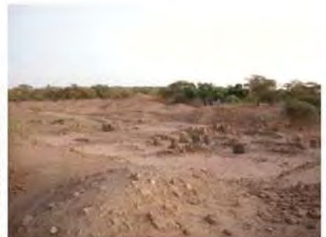
DSCN3973.JPG, Inappropriate Dumping of Excavation Spoils, Inappropriate/Inexistent Site Drainage, Royal City
