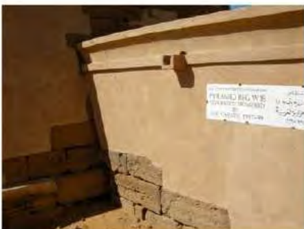
DSCN3827.JPG, Failure of Past Repair Work, Southern Cemetery
