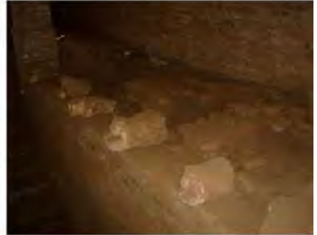
DSC06246.JPG, Inappropriate/Inexistent Site Drainage, Degradation of Stone/Masonry Elements, Royal City
