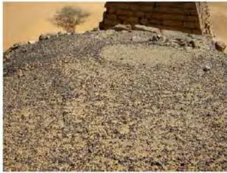
DSCN3849.JPG, Structural Deterioration of Pyramids, Southern Cemetery
