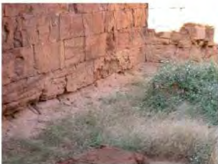
DSCN4026.JPG, Lion Temple B300 - Naqaa, Naqaa, Vegetation Damage, Degradation of Stone/Masonry Elements, Inappropriate/ Inexistent Site Drainage
