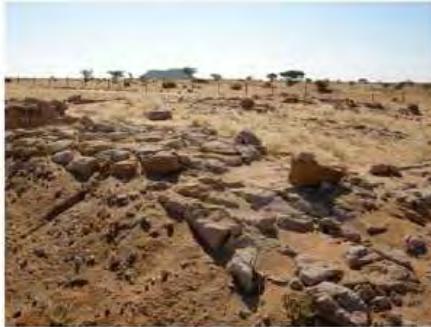
DSCN4083.JPG, Naqaa, Temple B200, Structural Instability of Walls/Collapse of Archaeological Features, Degradation of Stone/Masonry Elements, Inappropriate/Inexistent Site Drainage
