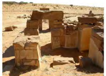
DSCN4119.JPG, Naqaa, Amun Temple, Exposure and Deterioration of Ancient Plasters, Inappropriate/Inexistent Site Drainage
