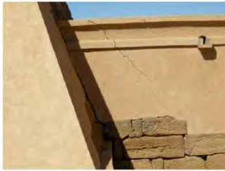
DSCN3831.JPG, Failure of Past Repair Work, Southern Cemetery
