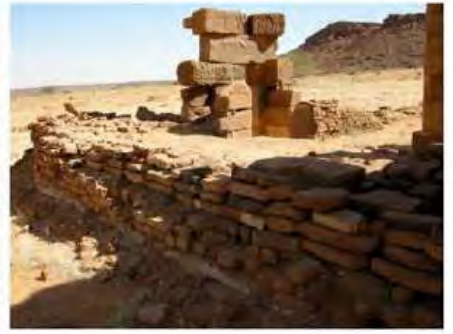
DSCN4095.JPG, Naqaa, Amun Temple, Structural Instability of Walls/Collapse of Archaeological Features, Exposure and Deterioration of Ancient Plasters, Degradation of Stone/Masonry Elements
