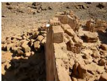
DSCN4158.JPG, Naqaa, Temple F, Structural Instability of Walls/Collapse of Archaeological Features, Structural Instability of Walls/Collapse of Archaeological Features
