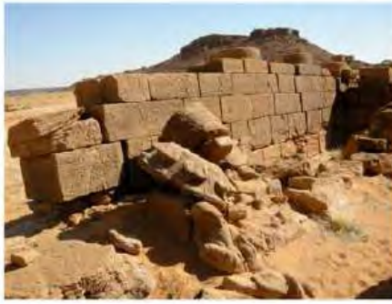
DSCN4083.JPG, Naqaa, Amun Temple, Structural Instability of Walls/Collapse of Archaeological Features, Inappropriate/Inexistent Site Drainage, Degradation of Stone/Masonry Elements
