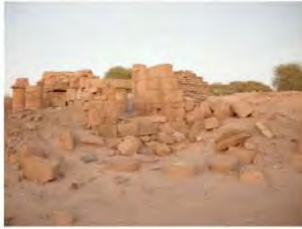
DSCN3991.JPG, Structural Instability of Walls/Collapse of Archaeological Features, Inappropriate Dumping of Excavation Spoils, Inappropriate/Inexistent Site Drainage, Royal City
