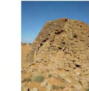
DSCN3863.JPG, Structural Deterioration of Pyramids, Southern Cemetery
