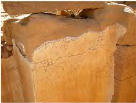
DSCN4115.JPG, Naqaa, Amun Temple, Exposure and Deterioration of Ancient Plasters
