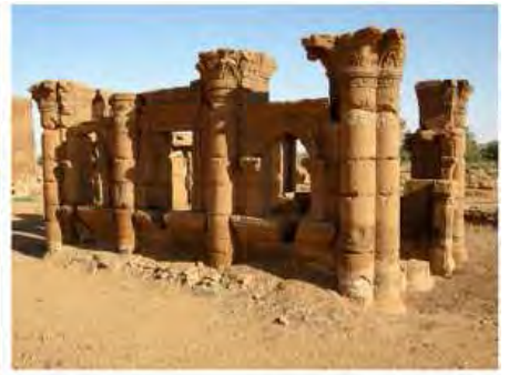
DSCN3998.JPG, The Kiosk - Naqaa, Naqaa, Degradation of Stone/ Masonry Elements, Inappropriate/Inexistent Site Drainage
