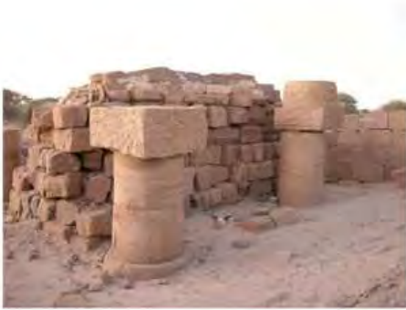
DSCN3980.JPG, Structural Instability of Walls/Collapse of Archaeological Features, Inappropriate Dumping of Excavation Spoils, Inappropriate/Inexistent Site Drainage, Royal City
