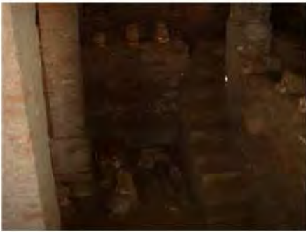
DSC06258.JPG, Inappropriate/Inexistent Site Drainage, Royal City
