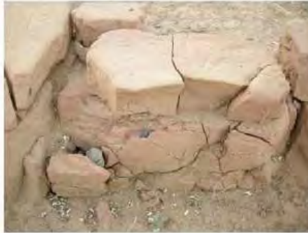
DSCN3933.JPG, Degradation of Stone/Masonry Elements, Structural Instability of Walls/Collapse of Archaeological Features, Royal City
