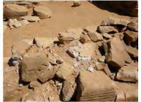
DSCN4178.JPG, Musawwarat - Great Enclosure, Structural Instability of Walls/Collapse of Archaeological Features, Structural Instability of Walls/Collapse of Archaeological Features, Restoration Works
