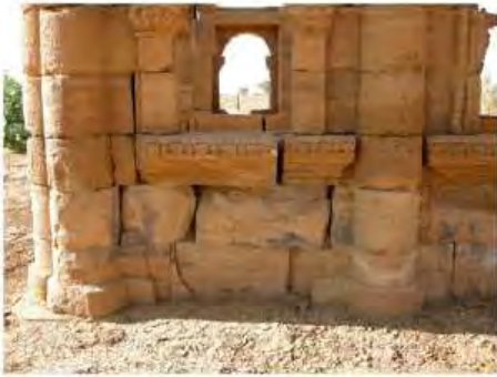
DSCN4015.JPG, The Kiosk - Naqaa, Naqaa, Degradation of Stone/ Masonry Elements, Inappropriate/Inexistent Site Drainage
