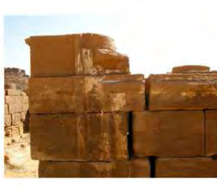
DSCN4082.JPG, Naqaa, Amun Temple, Exposure and Deterioration of Ancient Plasters
