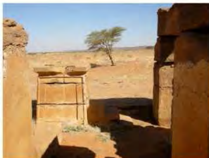
DSCN4112.JPG, Naqaa, Amun Temple, Exposure and Deterioration of Ancient Plasters, Inappropriate/Inexistent Site Drainage
