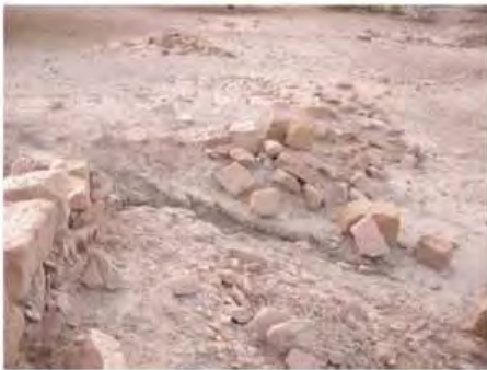
DSCN3983.JPG, Structural Instability of Walls/Collapse of Archaeological Features, Inappropriate Dumping of Excavation Spoils, Inappropriate/Inexistent Site Drainage, Royal City
