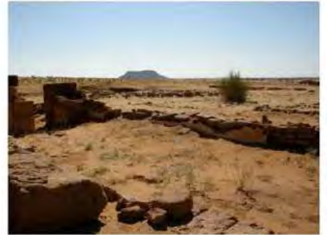
DSCN4108.JPG, Naqaa, Amun Temple, Exposure and Deterioration of Ancient Plasters, Structural Instability of Walls/ Collapse of Archaeological Features
