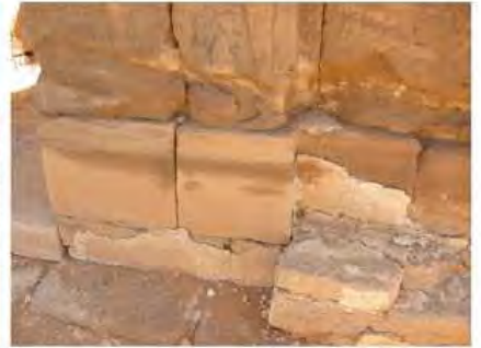
DSCN4092.JPG, Naqaa, Amun Temple, Exposure and Deterioration of Ancient Plasters, Degradation of Stone/Masonry Elements
