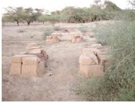
DSCN3930.JPG, Inappropriate/Inexistent Site Drainage, Degradation of Stone/Masonry Elements, Structural Instability of Walls/Collapse of Archaeological Features, Vegetation Damage, Royal City
