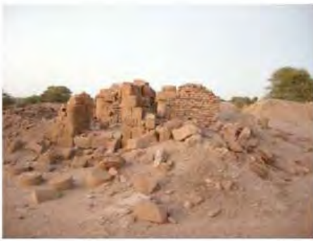
DSCN3977.JPG, Structural Instability of Walls/Collapse of Archaeological Features, Degradation of Stone/Masonry Elements, Inappropriate/Inexistent Site Drainage, Inappropriate Dumping of Excavation Spoils, Royal City
