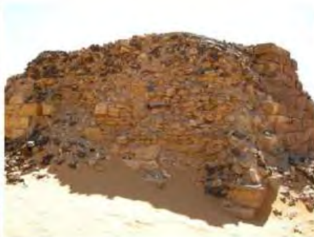
DSCN3739.JPG, Structural Deterioration of Pyramids, Northern Cemetery
