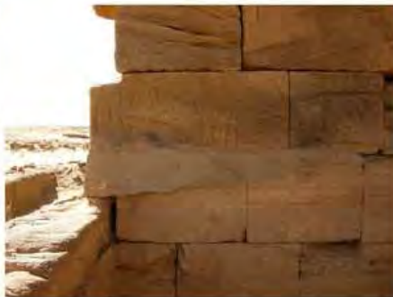
DSCN4128.JPG, Naqaa, Amun Temple, Unsympathetic Repair Work/Interventions, Degradation of Stone/Masonry Elements
