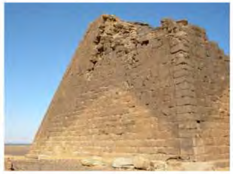
DSCN3758.JPG, Public Safety Hazard, Structural Deterioration of Pyramids, Northern Cemetery
