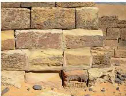
DSCN3717.JPG, Unsympathetic Repair Work/Interventions, Northern Cemetery
