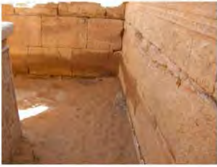
DSCN4127.JPG, Naqaa, Amun Temple, Inappropriate/Inexistent Site Drainage, Water Damage, Degradation of Stone/Masonry Elements
