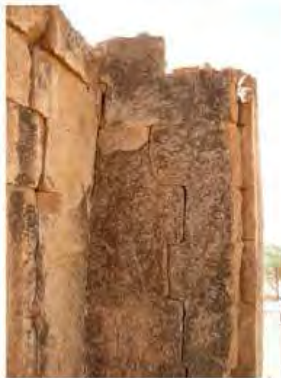
DSCN4150.JPG, Naqaa, Temple F, Structural Instability of Walls/Collapse of Archaeological Features, Structural Instability of Walls/Collapse of Archaeological Features, Exposure and Deterioration of Ancient Plasters
