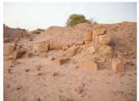
DSCN3976.JPG, Degradation of Stone/Masonry Elements, Structural Instability of Walls/Collapse of Archaeological Features, Inappropriate Dumping of Excavation Spoils, Inappropriate/Inexistent Site Drainage, Royal City
