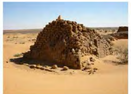
DSCN3841.JPG, Structural Deterioration of Pyramids, Southern Cemetery
