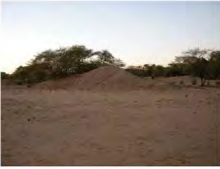
DSCN3929.JPG, Inappropriate Dumping of Excavation Spoils, Inappropriate/Inexistent Site Drainage, Royal City
