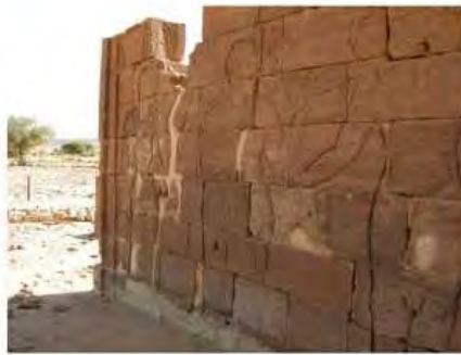
DSCN4036.JPG, Lion Temple B300 - Naqaa, Naqaa, Unsympathetic Repair Work/Interventions
