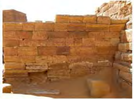
DSCN3737.JPG, Exposure and Deterioration of Ancient Plasters, Northern Cemetery
