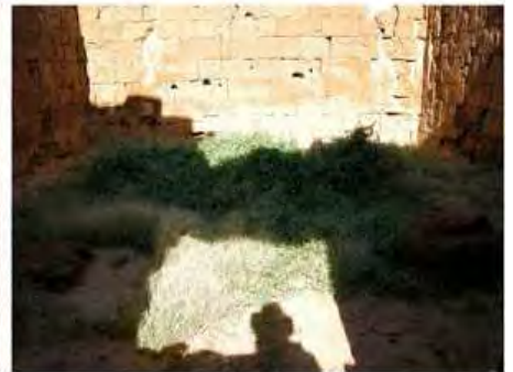
DSCN4023.JPG, Lion Temple B300 - Naqaa, Naqaa, Inappropriate/ Inexistent Site Drainage, Degradation of Stone/Masonry Elements, Vegetation Damage
