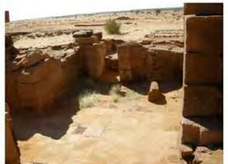
DSCN4122.JPG, Naqaa, Amun Temple, Vegetation Damage, Inappropriate/Inexistent Site Drainage, Degradation of Stone/Masonry Elements, Deterioration of Ancient Mud Structures
