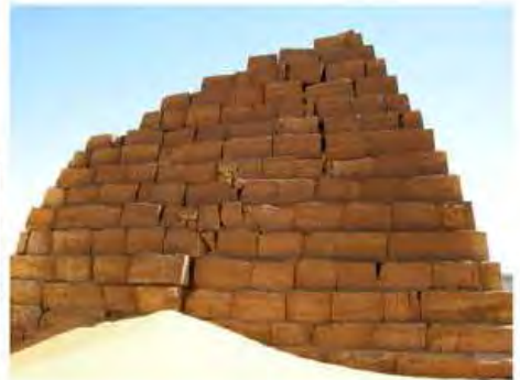
DSCN3740.JPG, Structural Deterioration of Pyramids, Northern Cemetery
