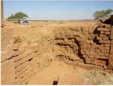
DSCN4109.JPG, Naqaa, Amun Temple, Deterioration of Ancient Mud Structures
