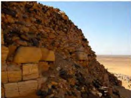
DSCN3738.JPG, Structural Deterioration of Pyramids, Northern Cemetery
