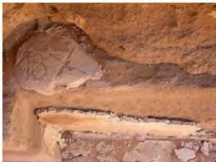
DSCN4093.JPG, Naqaa, Amun Temple, Exposure and Deterioration of Ancient Plasters, Degradation of Stone/Masonry Elements
