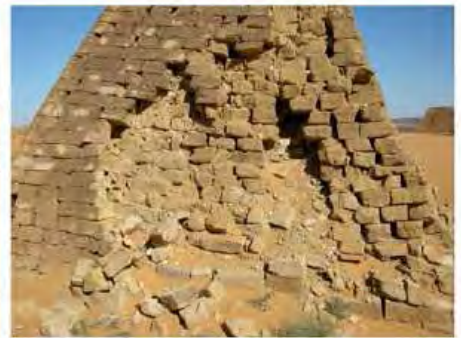
DSCN3886.JPG, Structural Deterioration of Pyramids, Southern Cemetery
