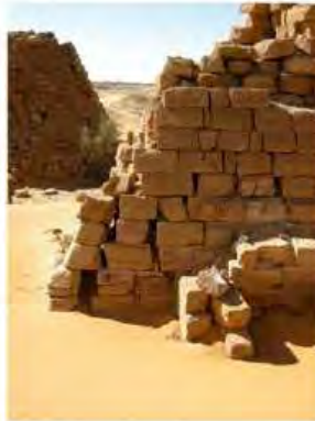
DSCN3858.JPG, Structural Deterioration of Pyramids, Southern Cemetery
