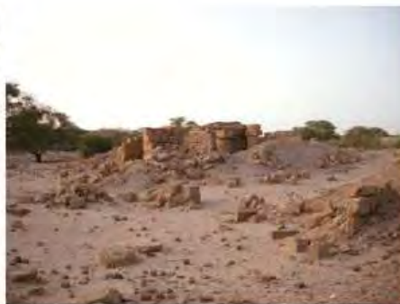
DSCN3975.JPG, Inappropriate Dumping of Excavation Spoils, Inappropriate/Inexistent Site Drainage, Structural Instability of Walls/ Collapse of Archaeological Features, Degradation of Stone/Masonry Elements, Royal City
