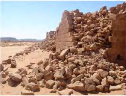
DSC06195.JPG, Musawwarat - Great Enclosure, Structural Instability of Walls/Collapse of Archaeological Features, Structural Instability of Walls/Collapse of Archaeological Features
