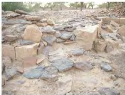
DSCN3948.JPG, Structural Instability of Walls/Collapse of Archaeological Features, Degradation of Stone/Masonry Elements, Royal City
