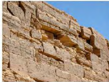
DSCN3712.JPG, Degradation of Stone/Masonry Elements, Northern Cemetery
