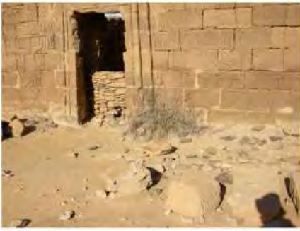
DSCN4020.JPG, Lion Temple B300 - Naqaa, Naqaa, Inaproprate/ Inexistent Site Drainage
