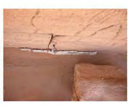
DSCN4085.JPG, Naqaa, Amun Temple, Exposure and Deterioration of Ancient Plasters
