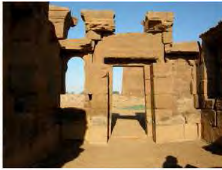
DSCN4010.JPG, The Kiosk - Naqaa, Naqaa, Degradation of Stone/ Masonry Elements, Inappropriate/Inexistent Site Drainage
