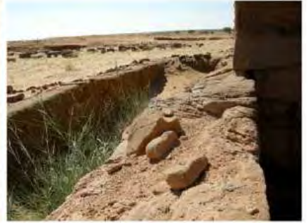
DSCN4131.JPG, Naqaa, Amun Temple, Degradation of Stone/Masonry Elements, Structural Instability of Walls/Collapse of Archaeological Features
