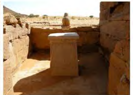
DSCN4126.JPG, Naqaa, Amun Temple, Water Damage, Inappropriate/Inexistent Site Drainage
