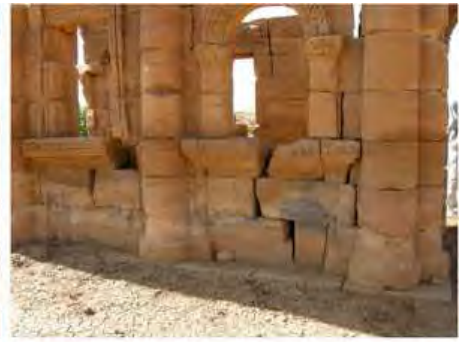
DSCN4014.JPG, The Kiosk - Naqaa, Naqaa, Degradation of Stone/ Masonry Elements, Inappropriate/Inexistent Site Drainage
