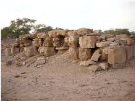
DSCN3956.JPG, Degradation of Stone/Masonry Elements, Structural Instability of Walls/Collapse of Archaeological Features, Royal City
