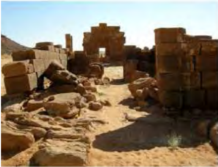
DSCN4080.JPG, Naqaa, Amun Temple, Exposure and Deterioration of Ancient Plasters, Structural Instability of Walls/ Collapse of Archaeological Features
