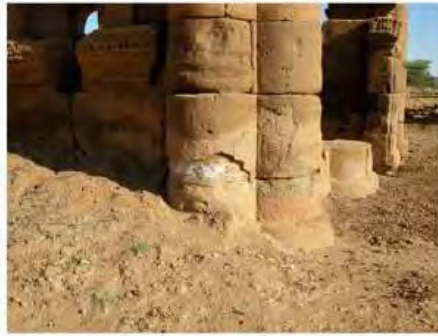
DSCN4000.JPG, The Kiosk - Naqaa, Naqaa, Degradation of Stone/ Masonry Elements, Inappropriate/Inexistent Site Drainage
