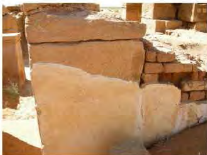
DSCN4117.JPG, Naqaa, Amun Temple, Exposure and Deterioration of Ancient Plasters, Deterioration of Ancient Mud Structures
