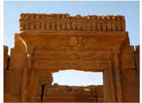
DSCN4016.JPG, The Kiosk - Naqaa, Naqaa, Structural Instability of Walls/Collapse of Archaeological Features
