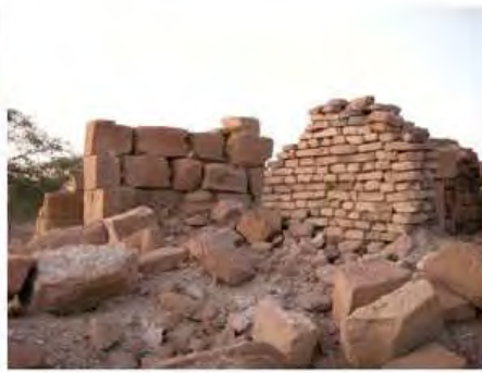
DSCN3978.JPG, Structural Instability of Walls/Collapse of Archaeological Features, Degradation of Stone/Masonry Elements, Inappropriate Dumping of Excavation Spoils, Inappropriate/Inexistent Site Drainage, Royal City
