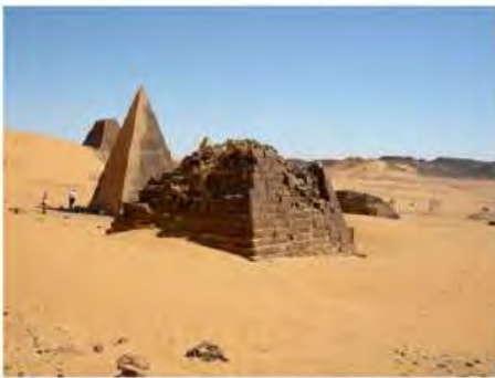
DSCN3762.JPG, Site Wide View, Structural Deterioration of Pyramids, Northern Cemetery
