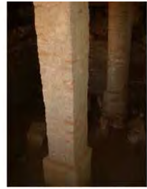
DSC06257.JPG, Inappropriate/Inexistent Site Drainage, Royal City
