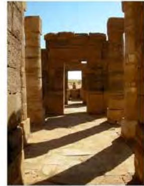
DSCN4087.JPG, Naqaa, Amun Temple, Degradation of Stone/ Masonry Elements
