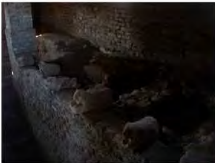
DSC06247.JPG, Inappropriate/Inexistent Site Drainage, Degradation of Stone/Masonry Elements, Royal City
