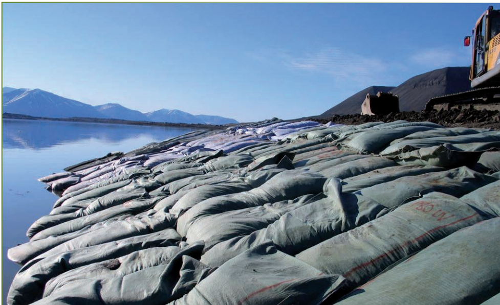
The testing of a new geosynthetic material for sandbagging coastal sites in danger of erosion (photo: SINTEF, Trondheim).
