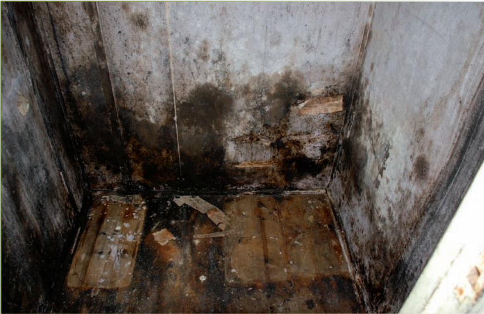
A bad case of mould and fungal growth in a protected building from 1957 in northeast Svalbard (photo: Susan Barr).
