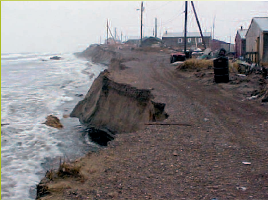
On the coast of western Alaska, village homes, ice cellars, water systems and infrastructures are being undermined by the sea, threatening the health of village residents (photo: Nome Nugget Newspaper).
