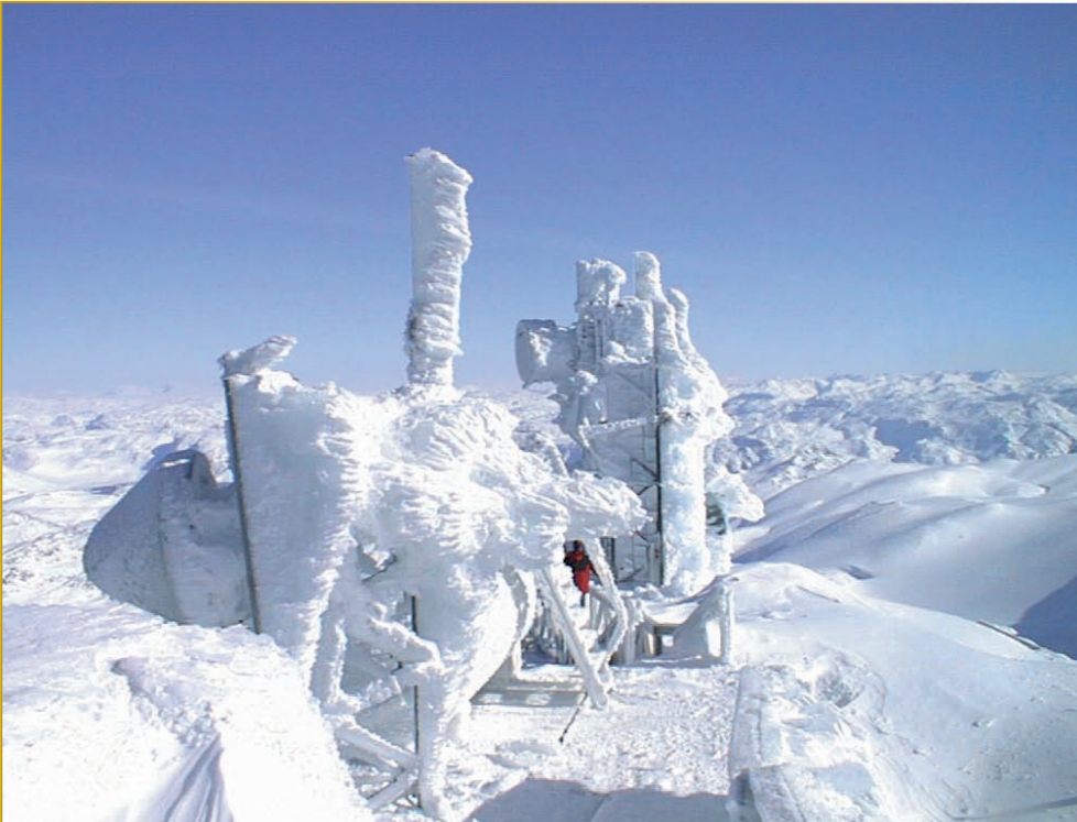
Iced over hill-top relay station in West Greenland (photo: Tele Greenland Ltd.).
