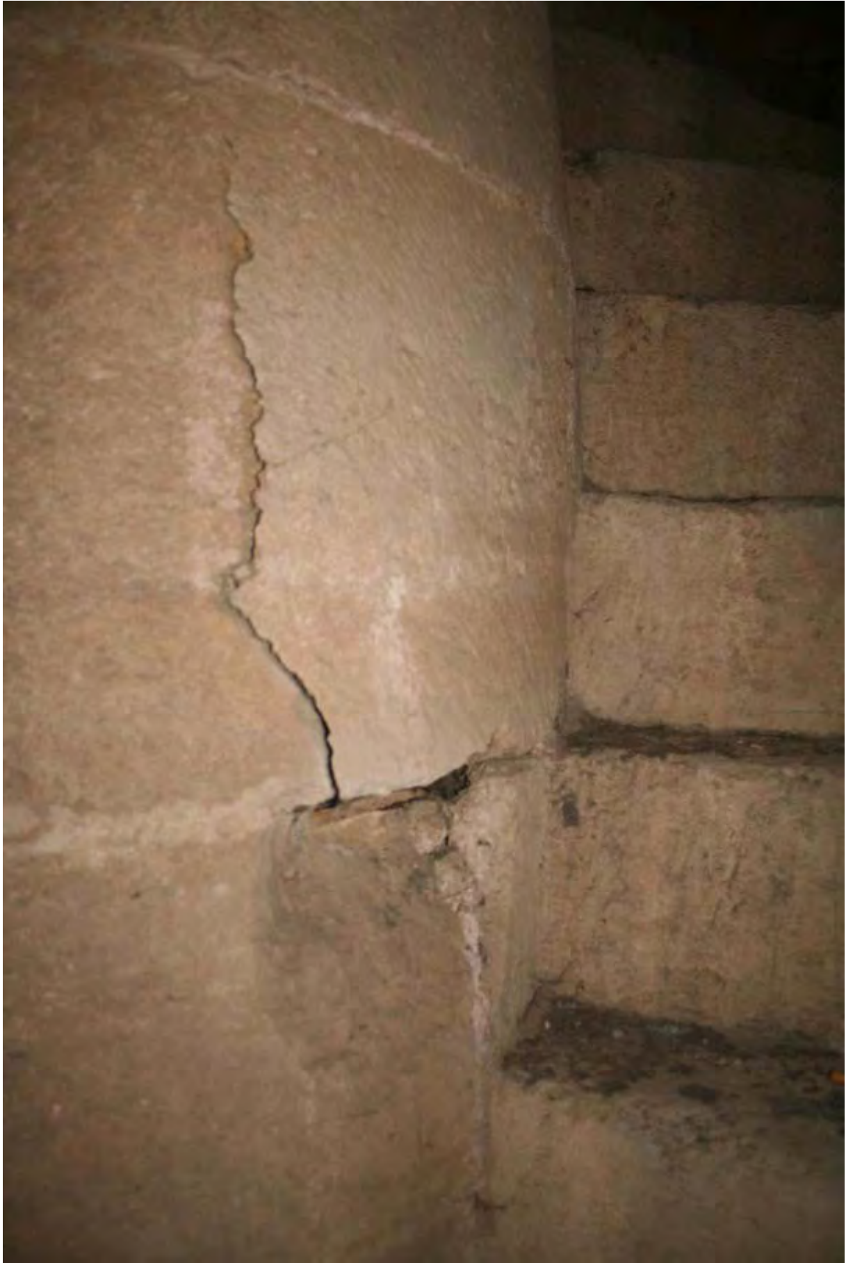
PHOTO 2- CONDITION OF MINARET STAIRS (2)
