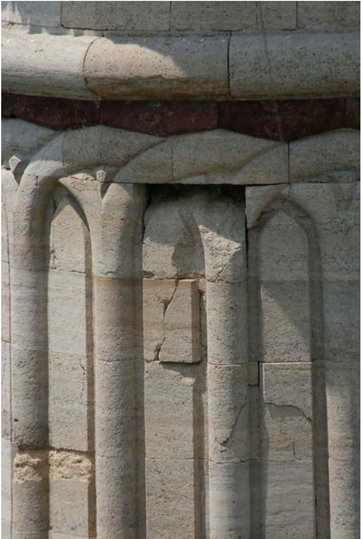
PHOTO 4- CORROSIONS ON MINARET SURFACE
