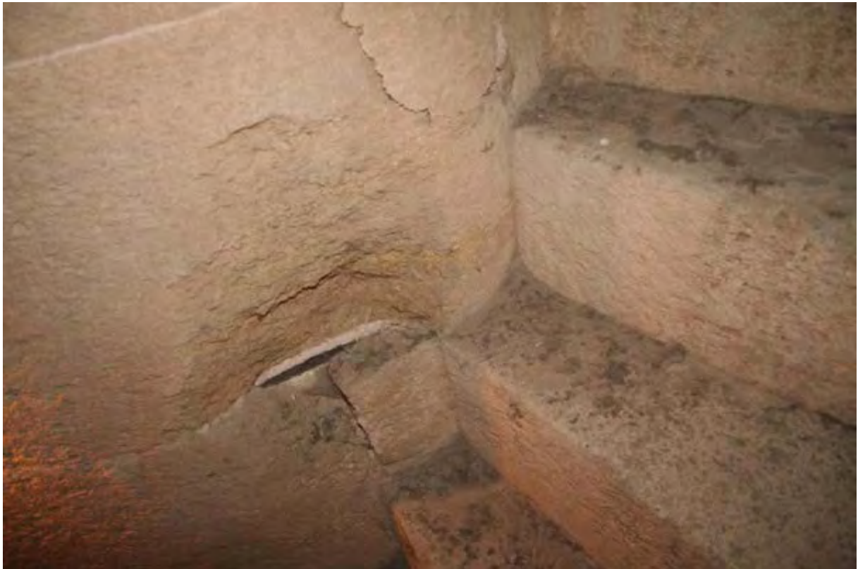
PHOTO 1- CONDITION OF MINARET STAIRS (1)
