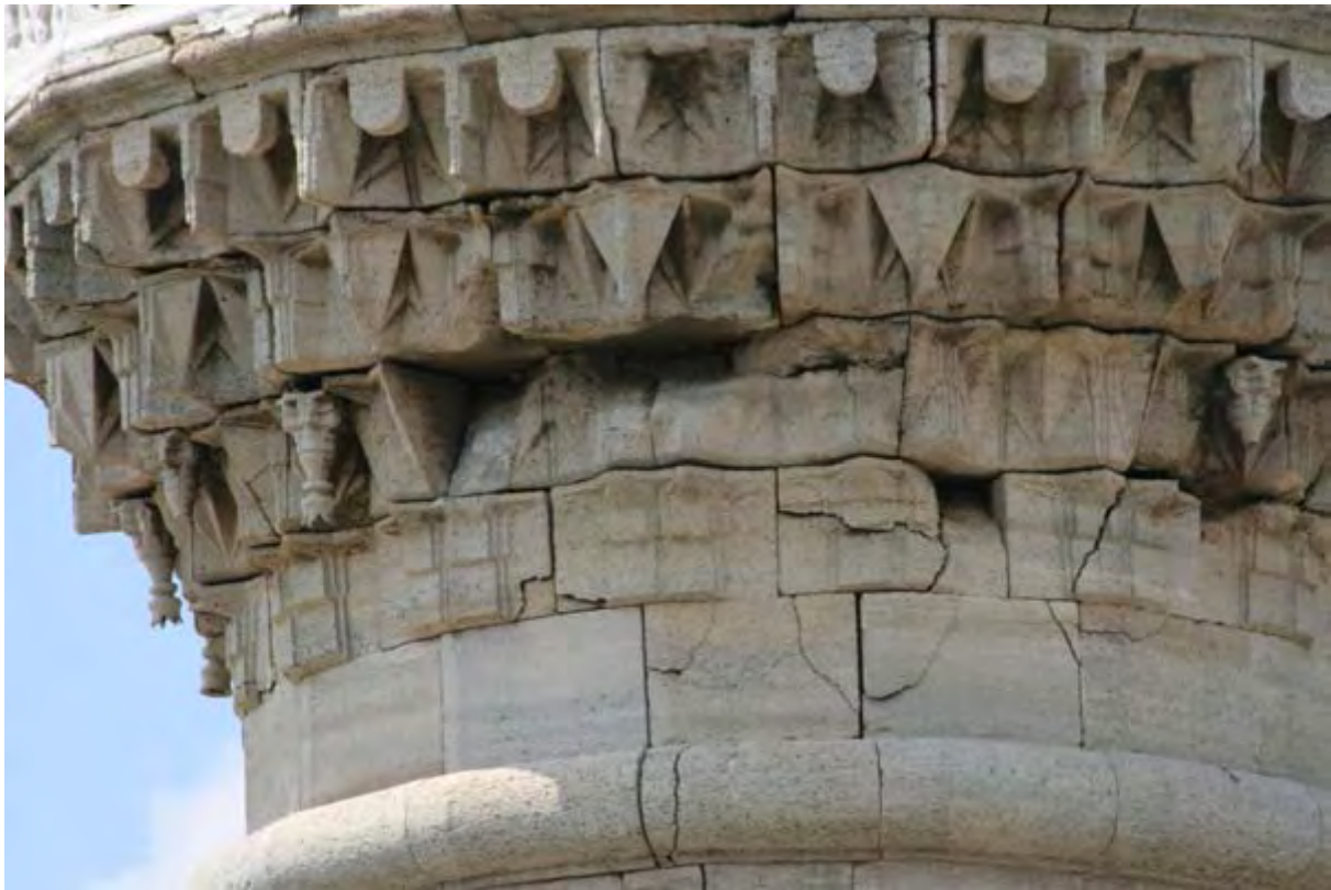
PHOTO 3- CORROSIONS ON MINARET MUKARNAS
