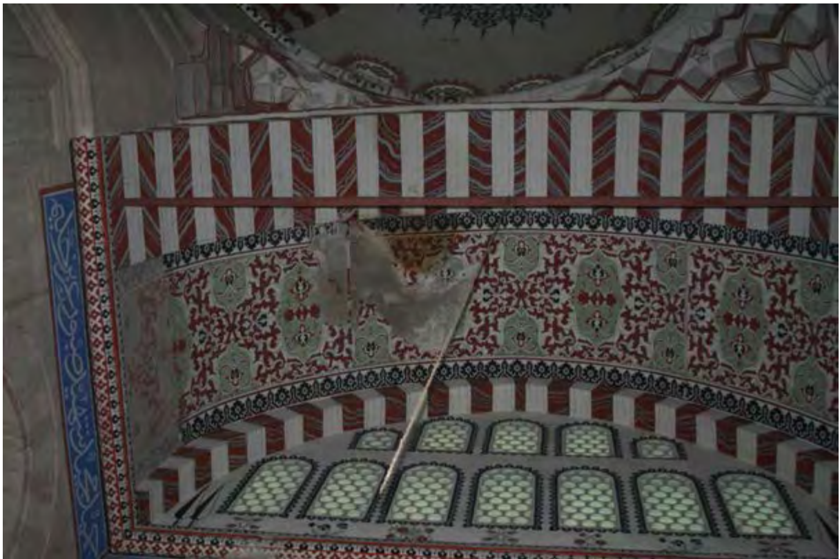
PHOTO 12- CORROSIONS ON FRESKS IN INNER PART
