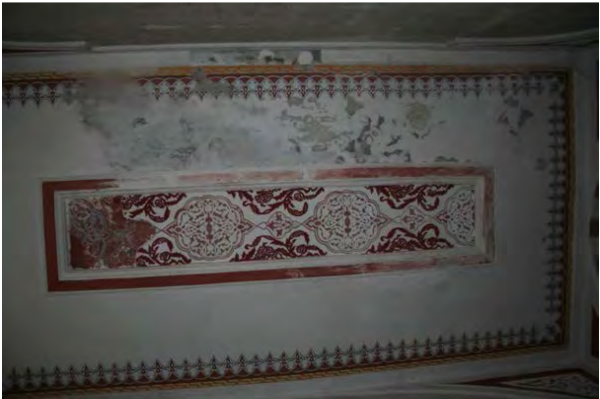
PHOTO 14- CORROSIONS ON GYPSUM WORKS INTERIOR
