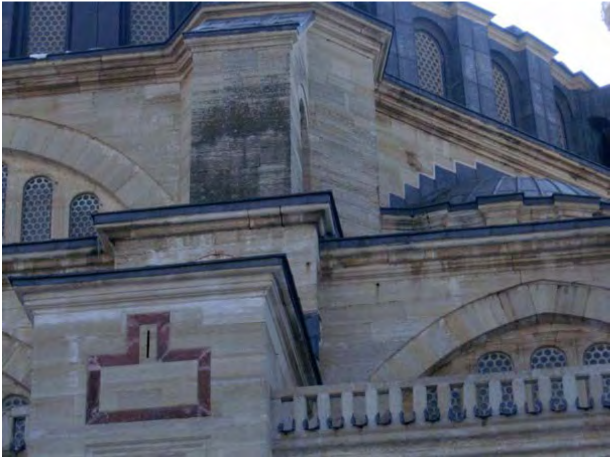
PHOTO 10- MOSSING ON SURFACES
