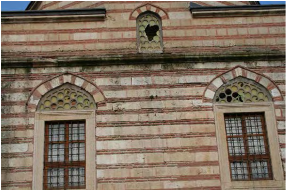
PHOTO 17- MOSSING ON FILLETS ON CORANIC SCHOOL
