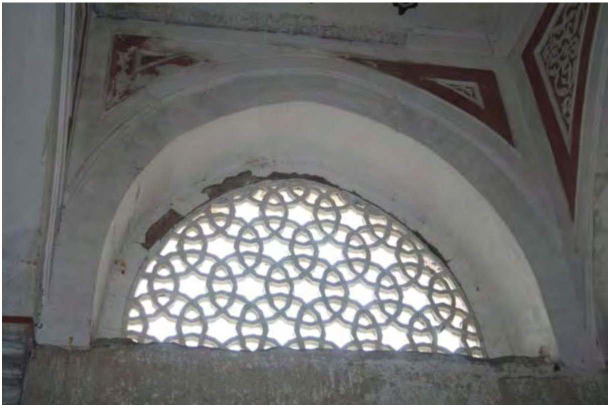
PHOTO 13- CORROSIONS ON GYPSUM WORKS IN INNER PART
