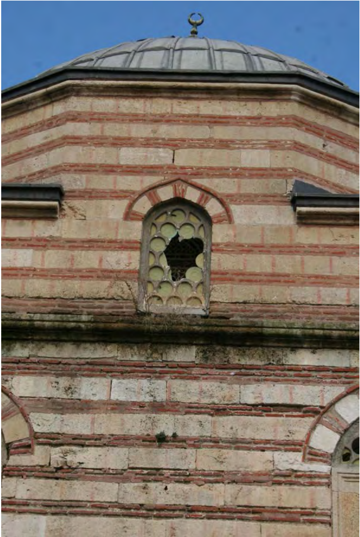
PHOTO 18- BROKEN GLASSES AT CORANIC SCHOOL
