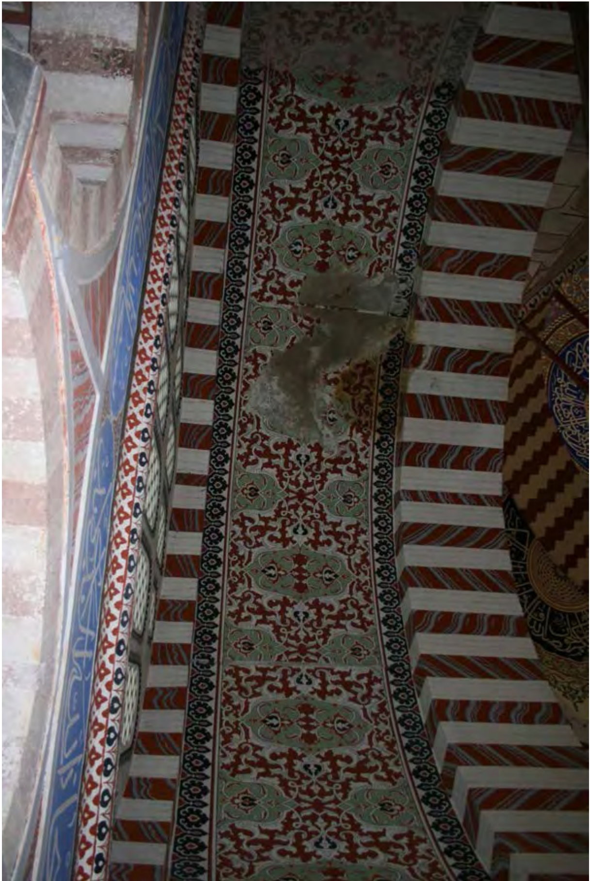
PHOTO 11- CORROSIONS ON FRESKS
