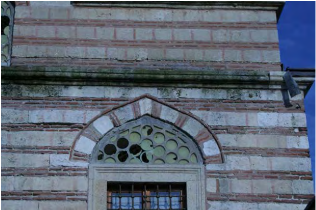
PHOTO 16- CORROSIONS ON FILLET AND BROKEN GLASSES OF CORANIC SCHOOL
