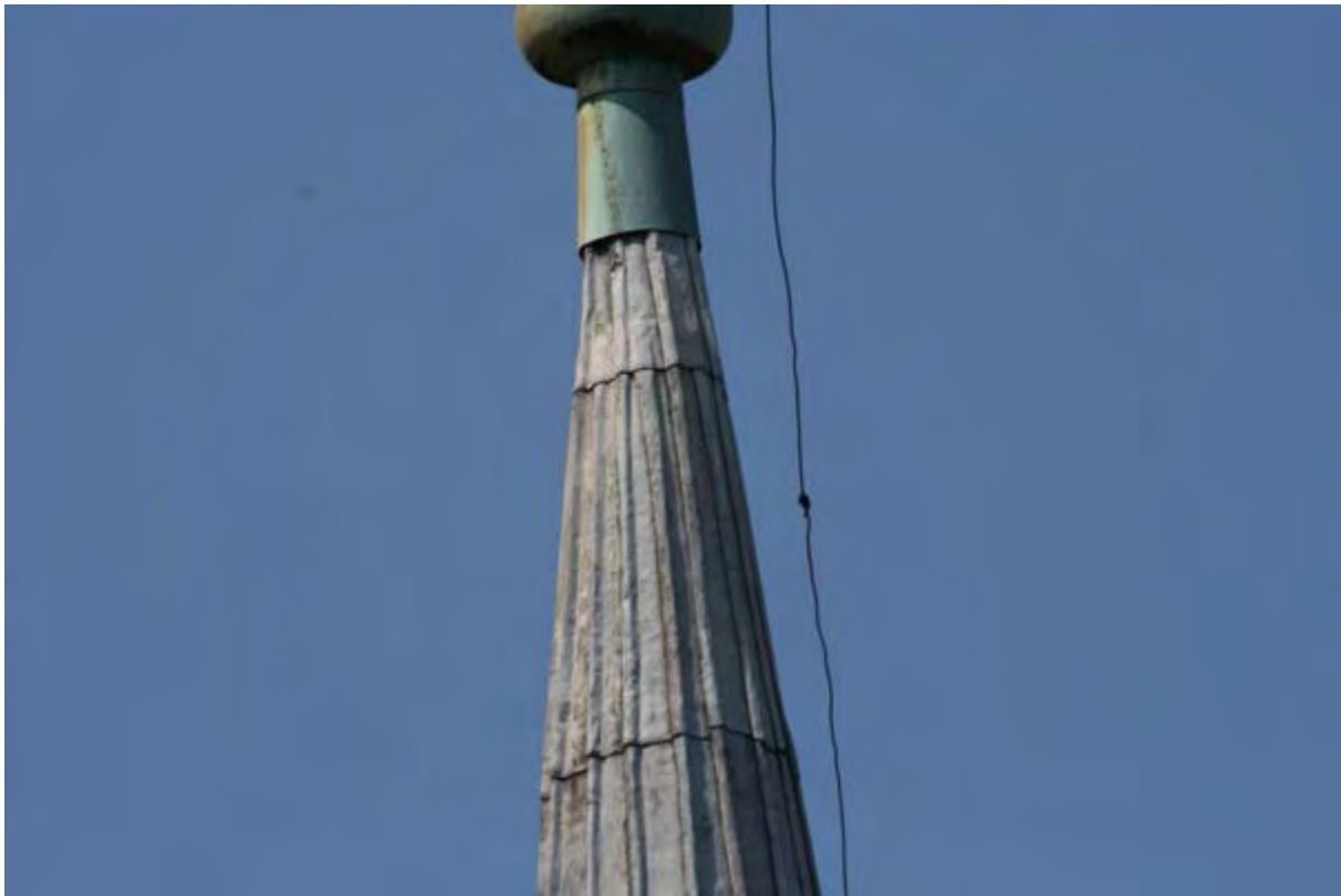
PHOTO 5- DETERIORATION ON LEADS OF SPIRES
